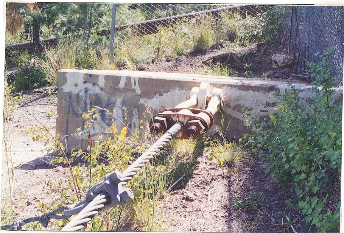
Peggy Sue Bridge (east end), detail of anchor inside fence, dir. ~E
