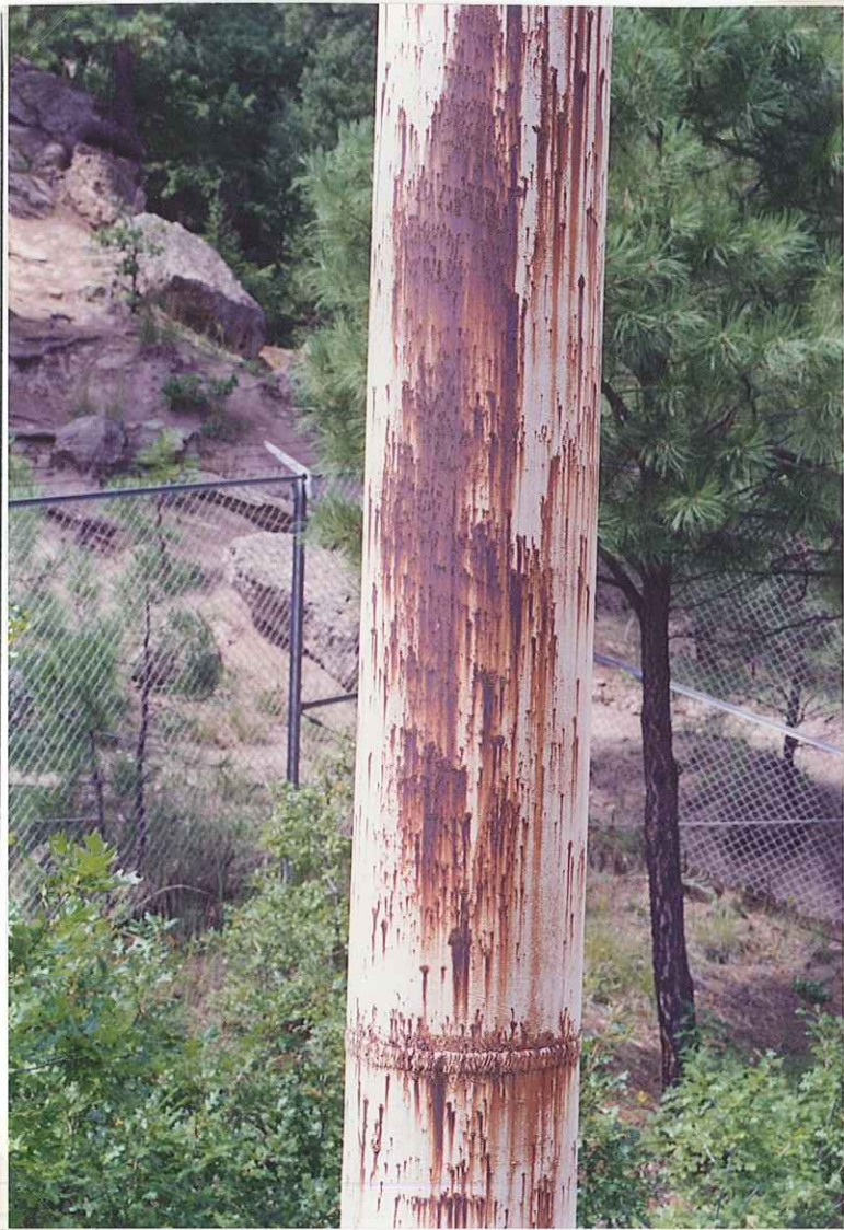
Peggy Sue Bridge, west tower detail showing rust, dir. ~W
