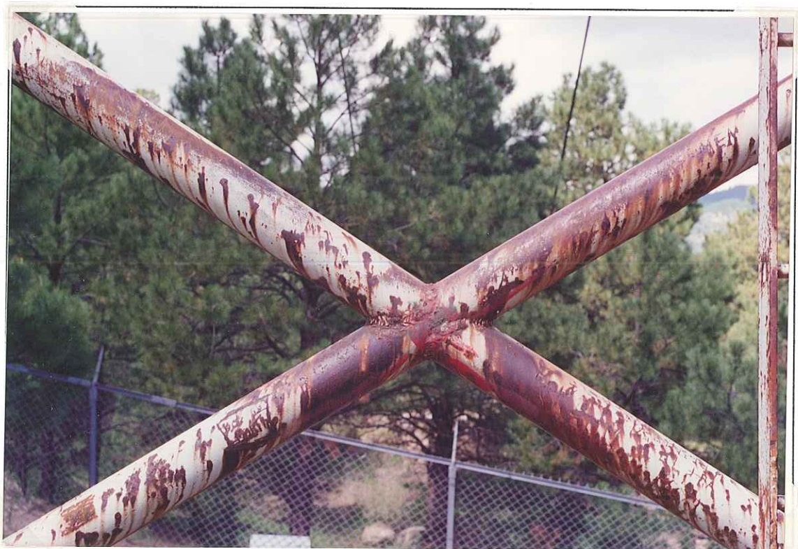
Peggy Sue Bridge, west tower detail showing rust, dir. ~W
