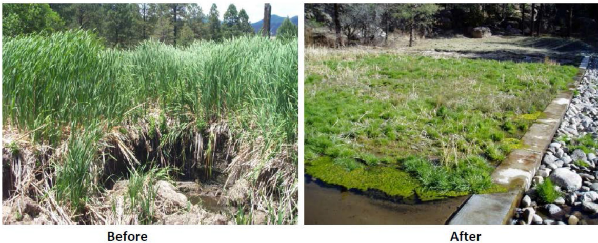
Figure 7-29 Gully erosion in 2007 (left photo) and the affected area in 2016 after installation of the grade-control structure (right photo) at the downstream end of the Sandia Canyon wetland
