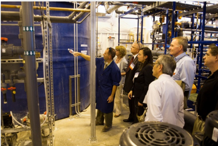
Community leaders tour the Sanitary Effluent Reclamation Facility (SERF) that recycles over 300 thousand gallons of sanitary wastewater a day to use in cooling super computers.
