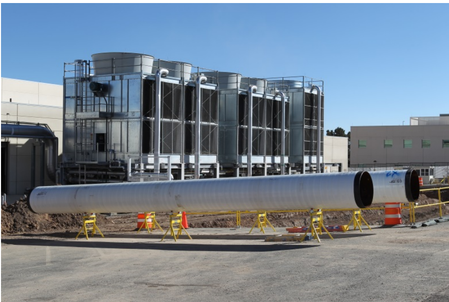
Major upgrades to the SCC support warm water cooling technology for the first phase of liquid supercomputing. Using warmer water requires less energy, thereby saving both energy and water.
