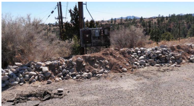
PT-SMA-2, Rock Berm, I00403120010 (photo ID 13420-1r)
