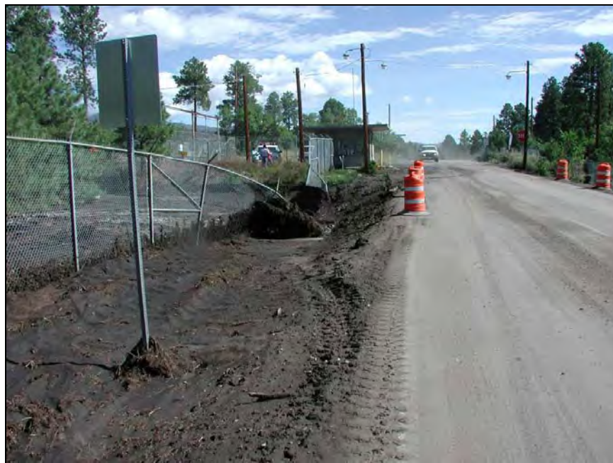
Photograph 42. Security fence at along Anchor Ranch Road damaged by flood event.
