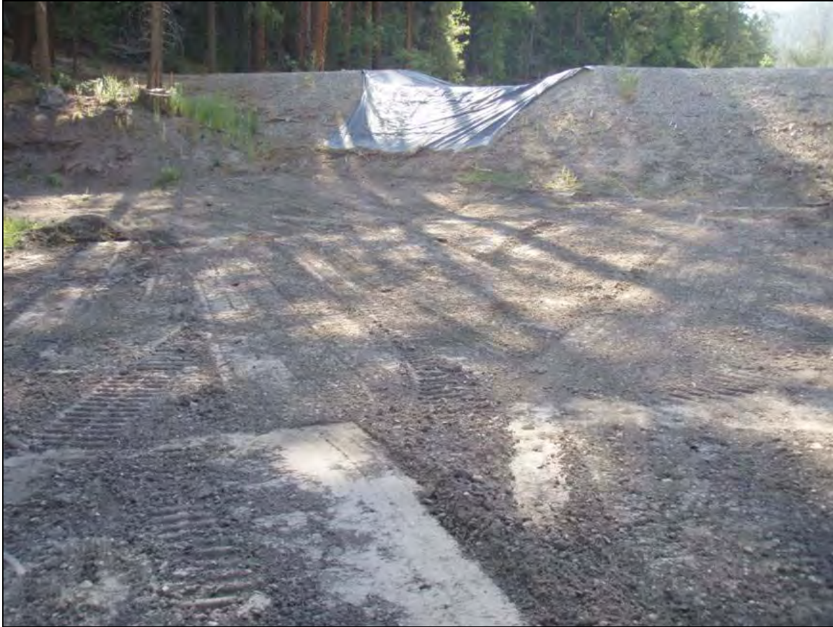
Photograph 11. Los Alamos Canyon retention basin.
