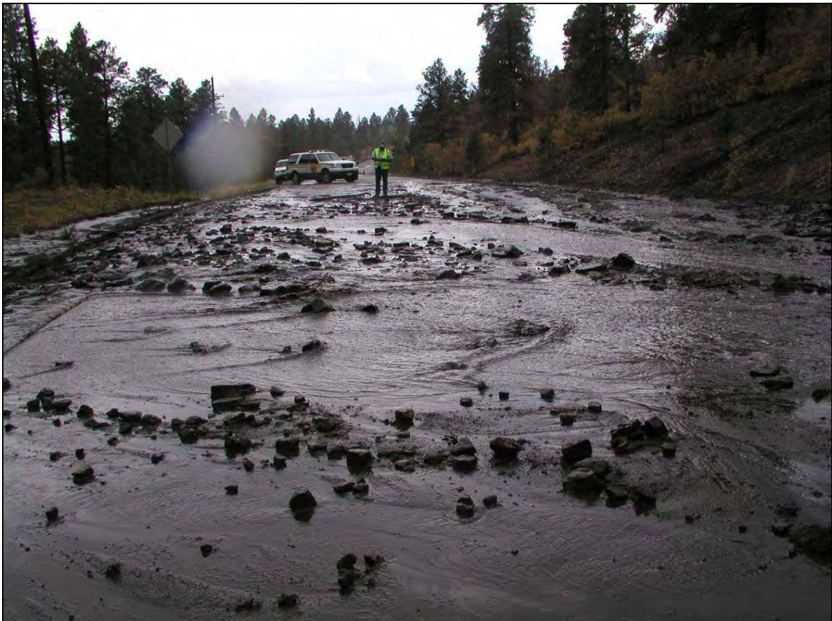
Photograph 36. Post-fire flooding effects on NM 501.
