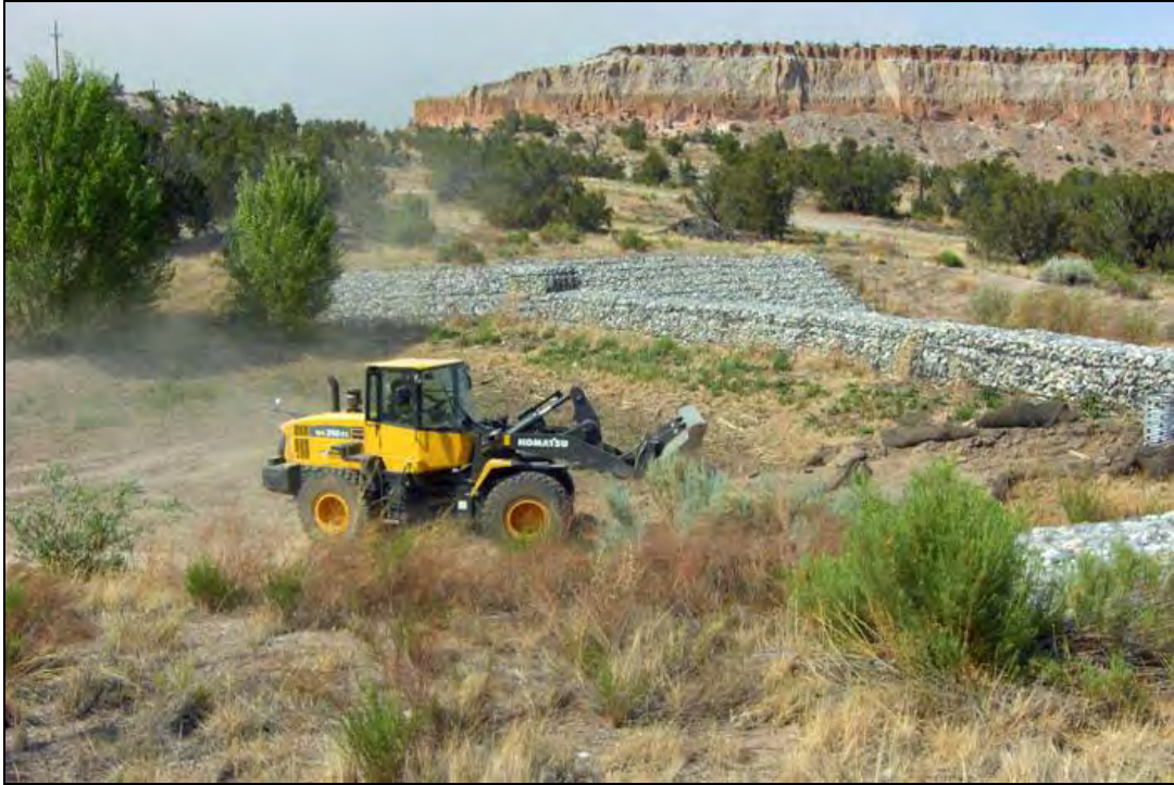
Photograph 8. Crews using heavy machinery to remove sediment from the Los Alamos Canyon Weir to restore its storage capacity.
