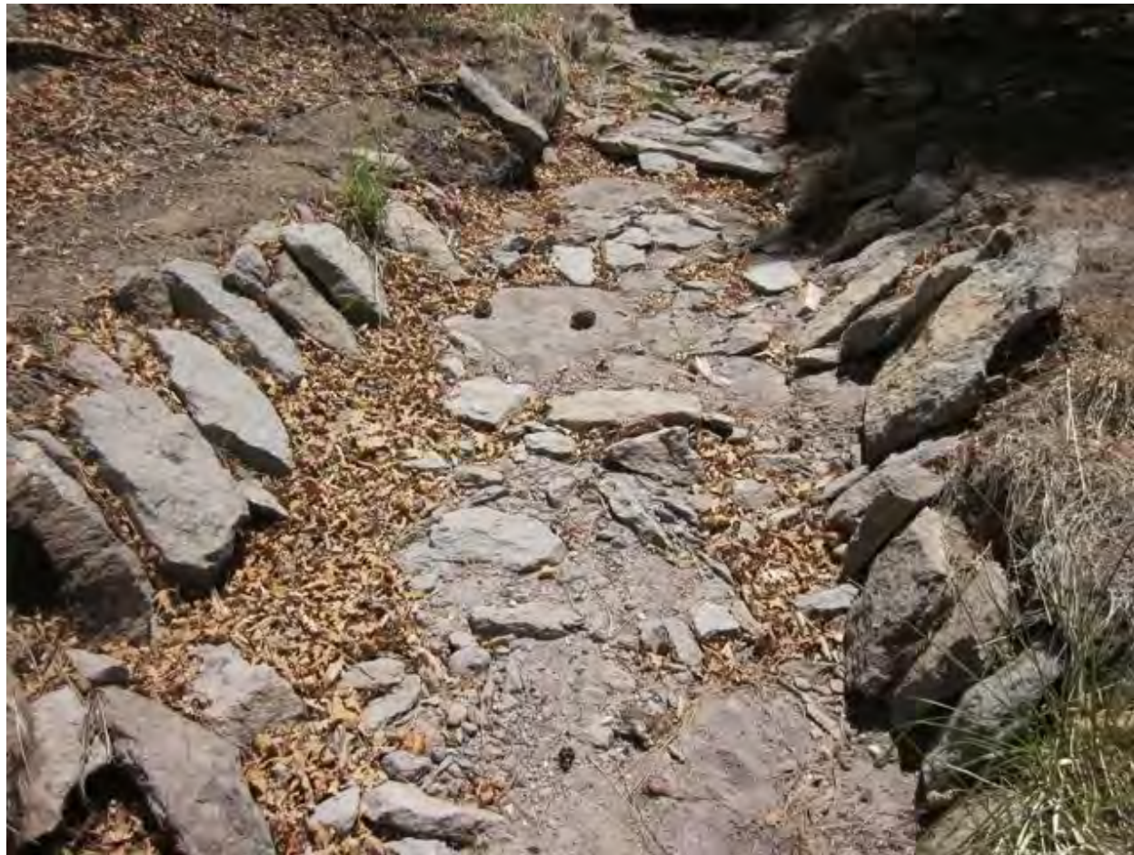
Figure 24 May 2011 photograph of rock armoring along stream banks in the south fork of Acid Canyon, looking upstream
