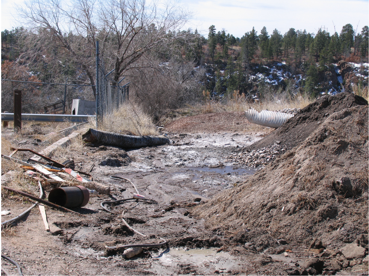
Figure 2 Runoff and debris in the south-central portion of former TA-32 near the canyon edge (March 2008)
