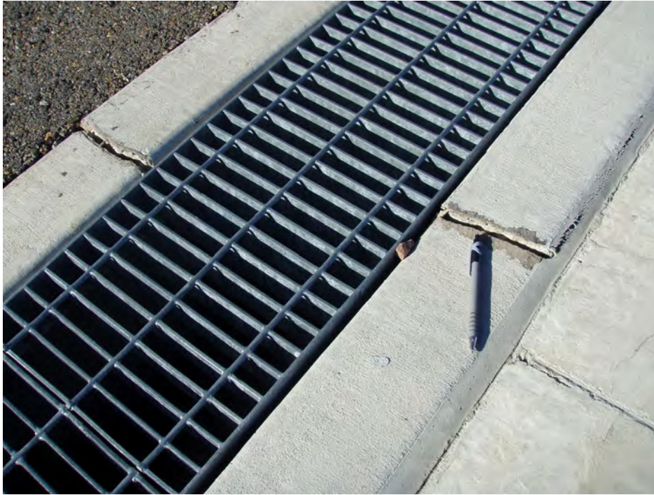
Figure 14 Crack across trench drain at hangar pad 1
