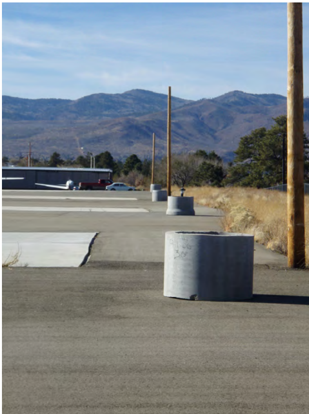
Figure 19 Gas vent locations, note missing risers and spinners
