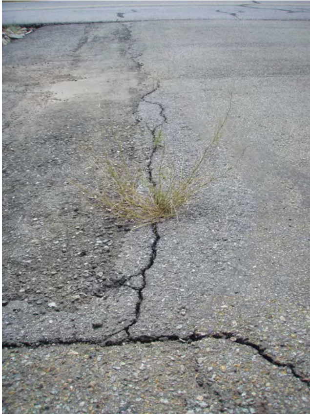
Figure 6 Vegetation growing within cracks of the MatCon pavement near the gravel drainage channel
