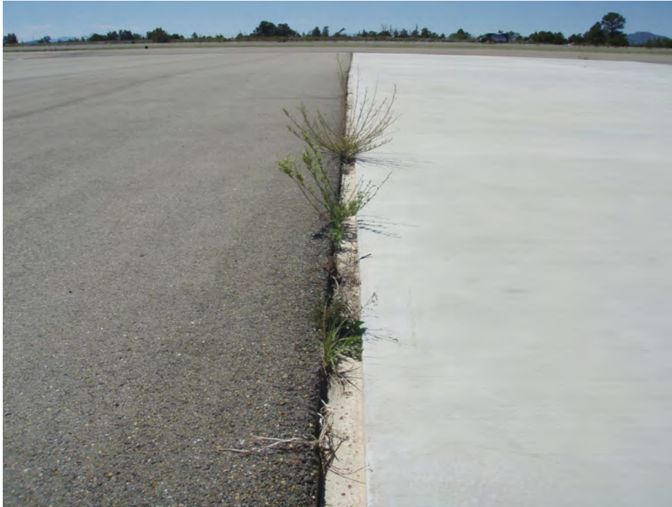
Figure 10 Vegetation growing between MatCon and hangar pad 4
