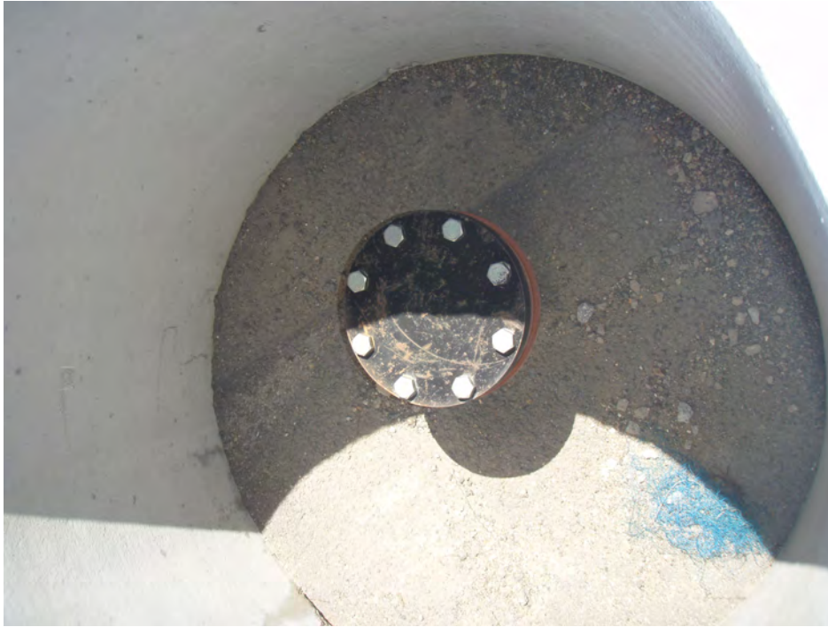
Figure 18 Gas vent with capping flange
