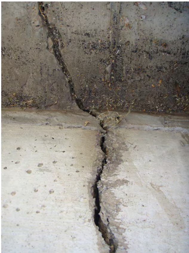
Figure 15 Crack across bottom and side of trench drain at hangar pad 1
