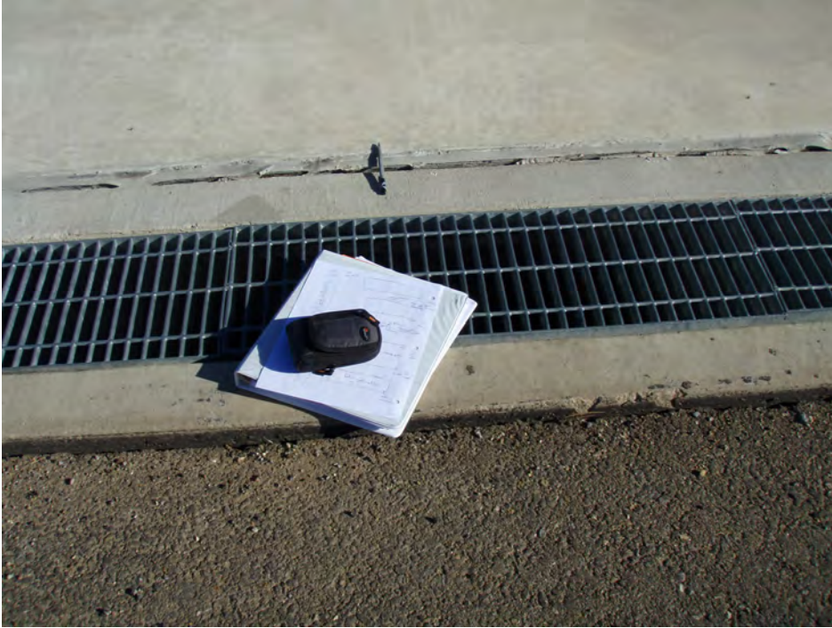
Figure 16 Separation between hangar pad and trench drain, note subsidence of MatCon pavement
