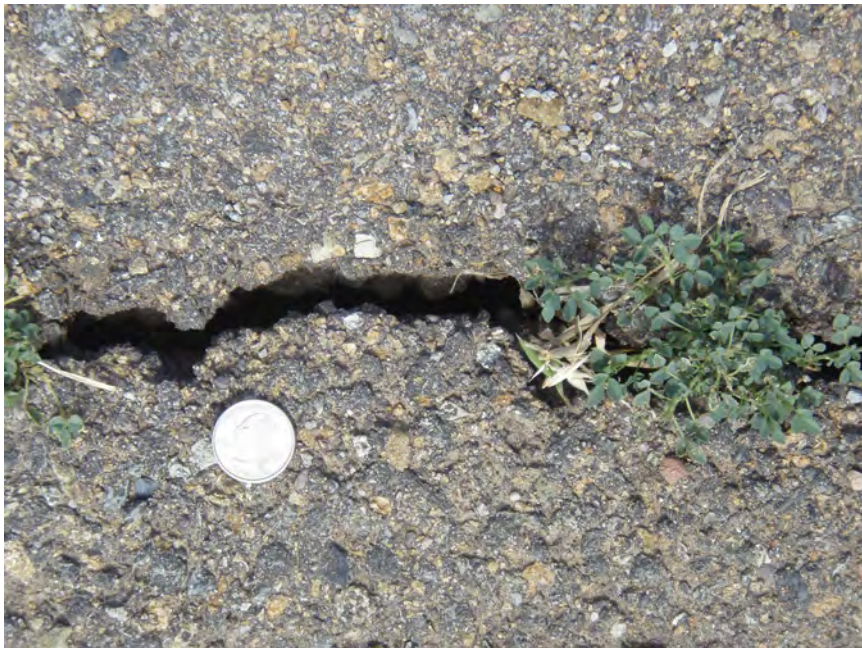
Figure 7 Vegetation growing in crack in MatCon pavement south of hangar pad 1
