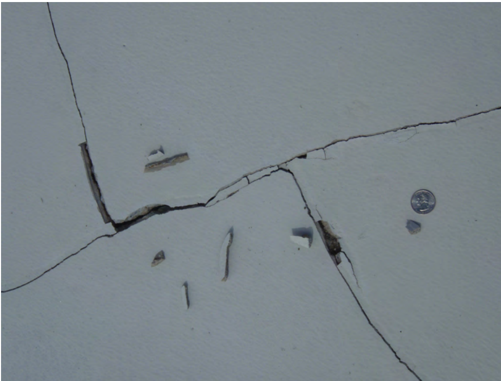
Figure 9 Typical cracking observed in hangar pads 1, 2, 3, and 4
