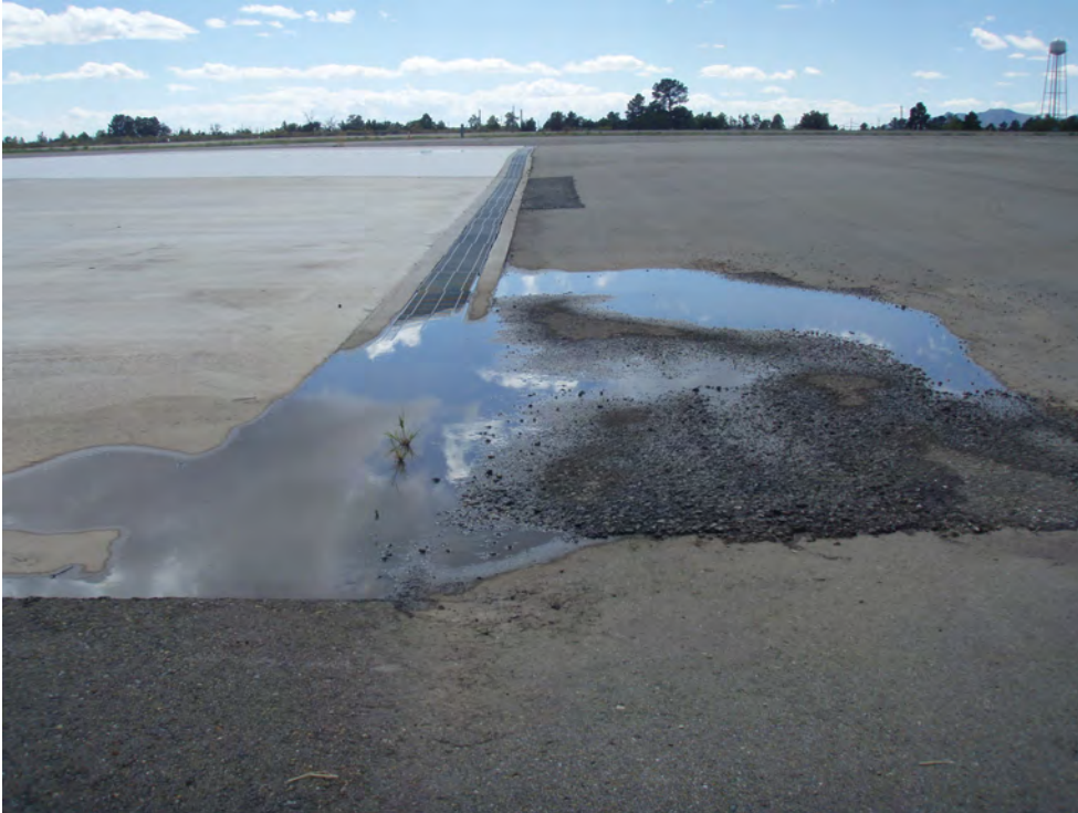
Figure 8 Ponding of water at northwest corner of hangar pad 3, note asphalt patches
