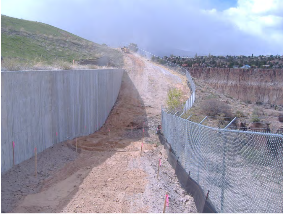
AREAS S, R, AND V-IMPORTING FILL MATERIAL TO BRING SURFACE TO REQUIRED GRADE
