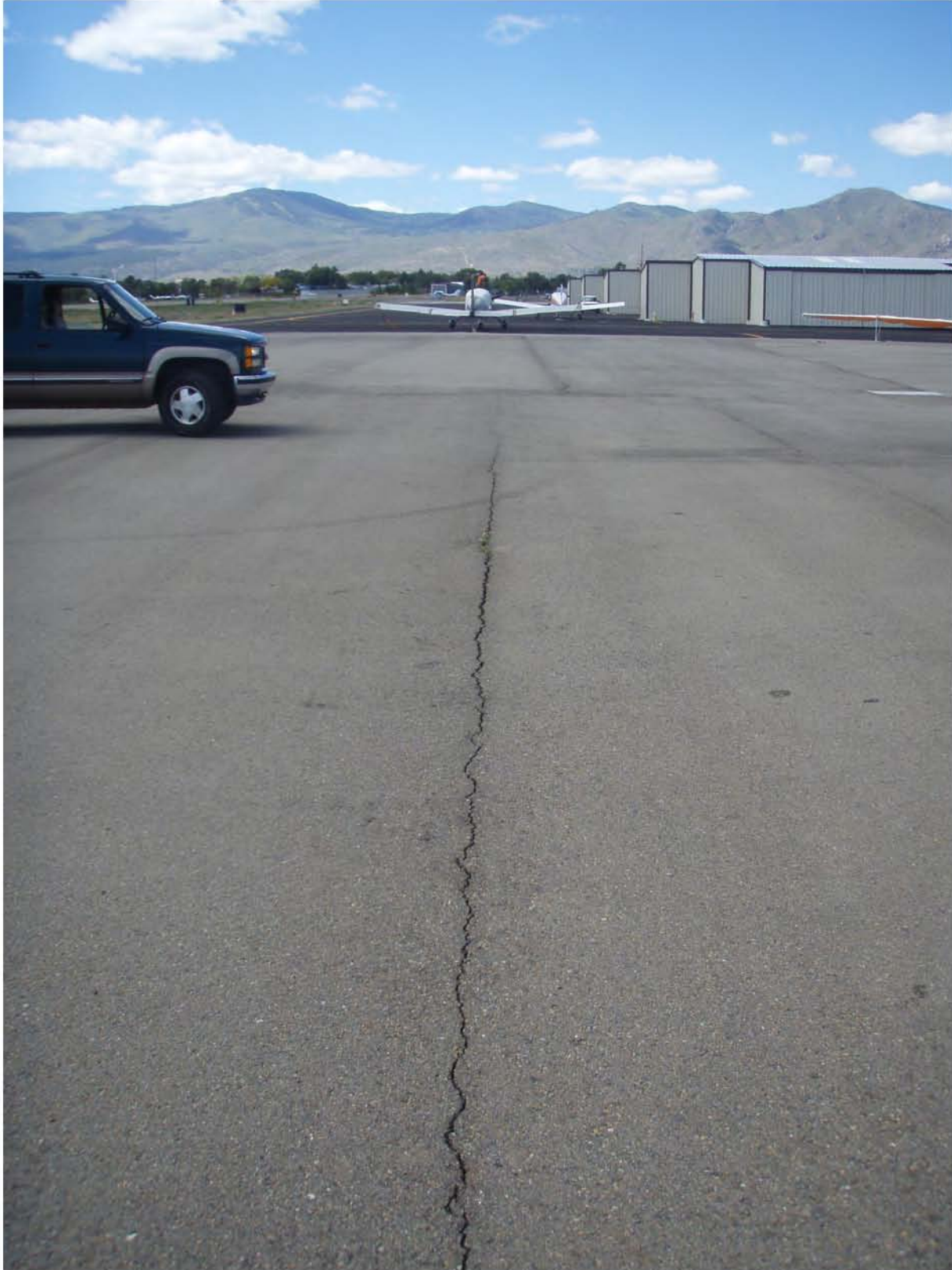
Figure 5 Typical crack in MatCon pavement, view to the west
