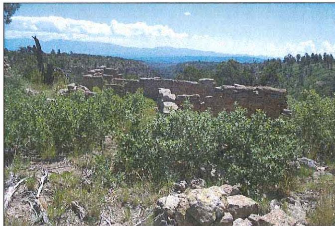
Figure 5. Southeastern corner of the eastern roomblock at Nake'muu (view southeast). Scrub oak is beginning to impact standing walls.
