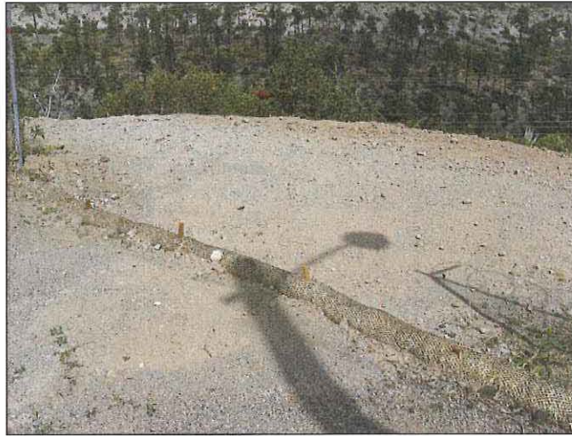
Site of septic tank removal in TA-46, note BMPs installed as per PR-ID comments.
