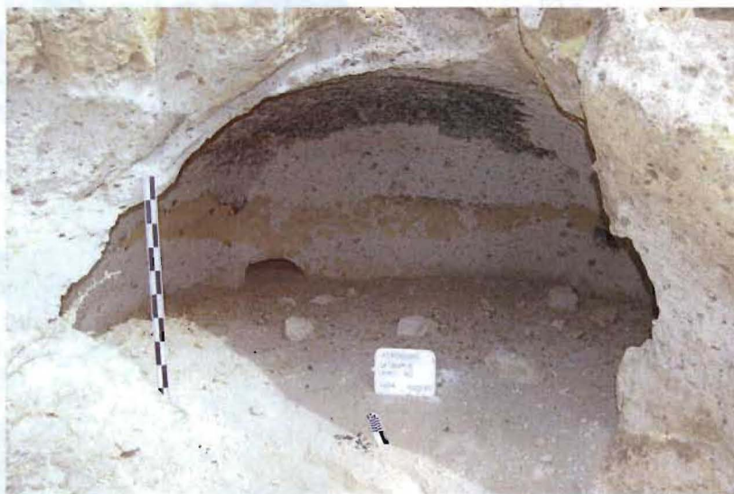
Figure 4. A cavate subject to erosion with spalling and deteriorating plaster and sooting.
