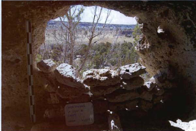
Figure 5. Cavate with stacked masonry blocks deemed fragile by assessors.
