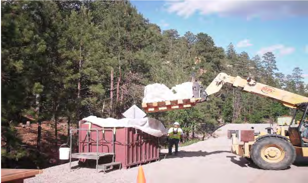
Bags of excavated media being loaded into waste box in the bottom of Los Alamos Canyon
