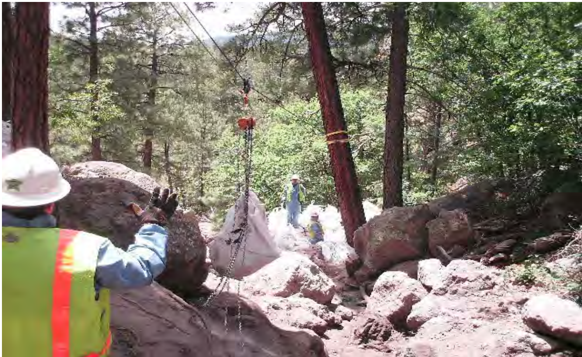
Transfer of waste bags from hillside drainage to canyon bottom via zip line
