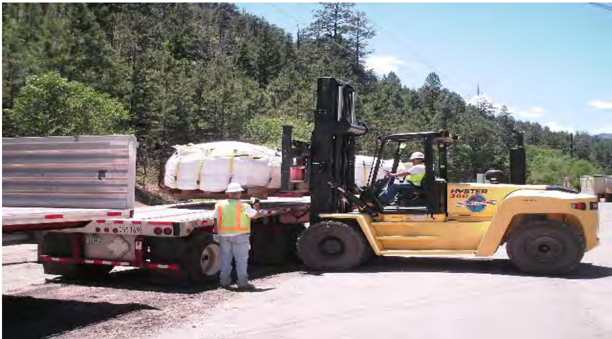
Bags of excavated media being loaded onto trucks for transport to Energy Solutions in Clive, Utah
