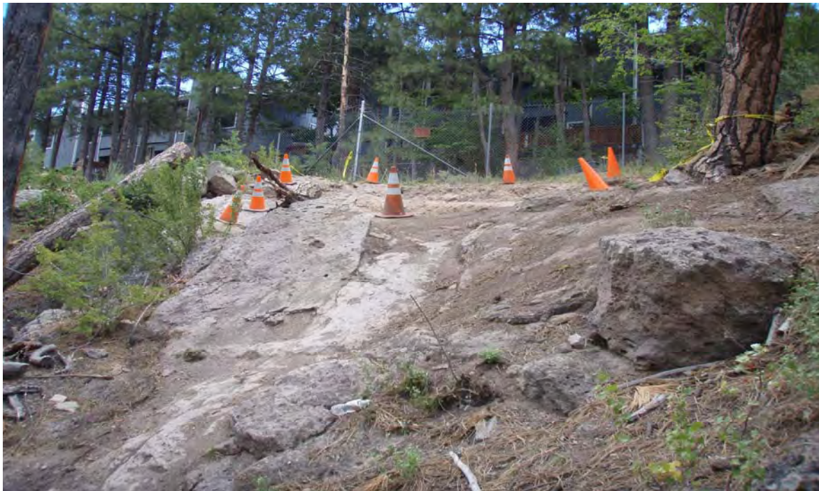
Excavated area in lower portion of Area 1 directly below the SWMU 01-001(f) outfall
