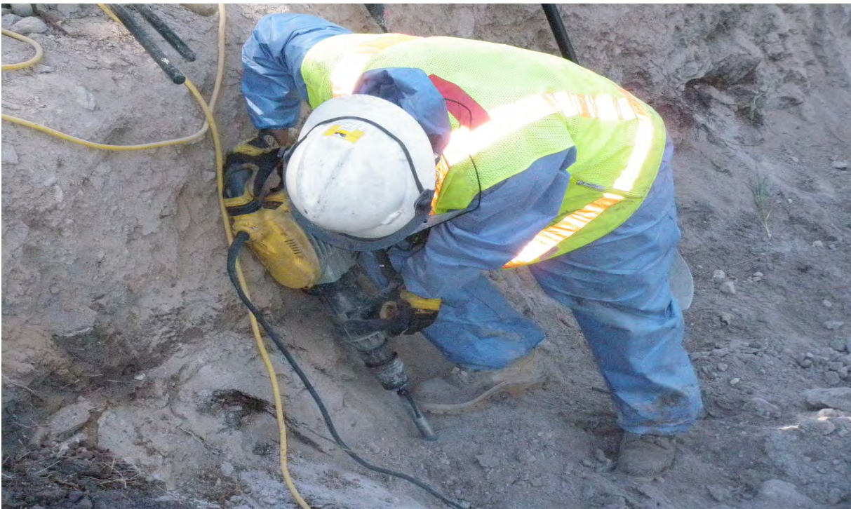
Use of air hammers to remove contaminated media from drainage below the SWMU 01-001(f) outfall
