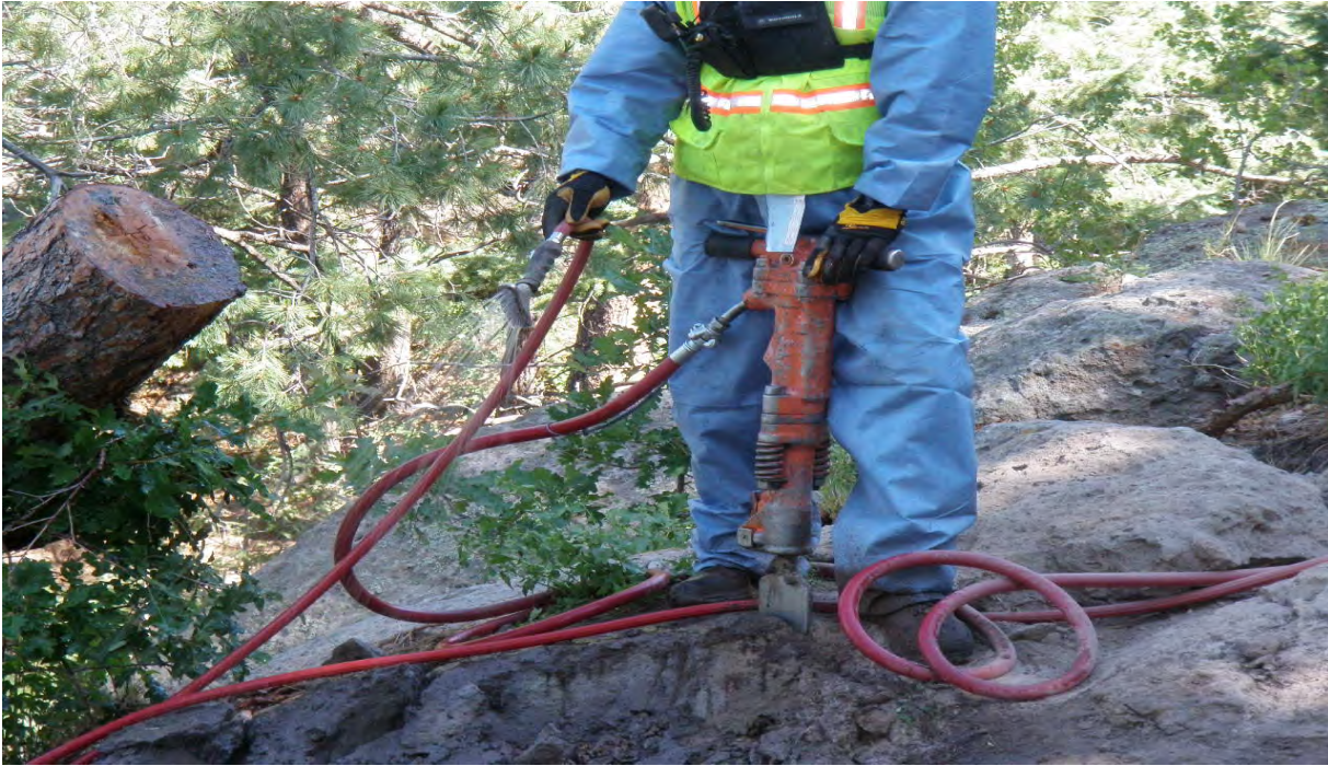
Use of air hammers to remove contaminated media from drainage below the SWMU 01-001(f) outfall
