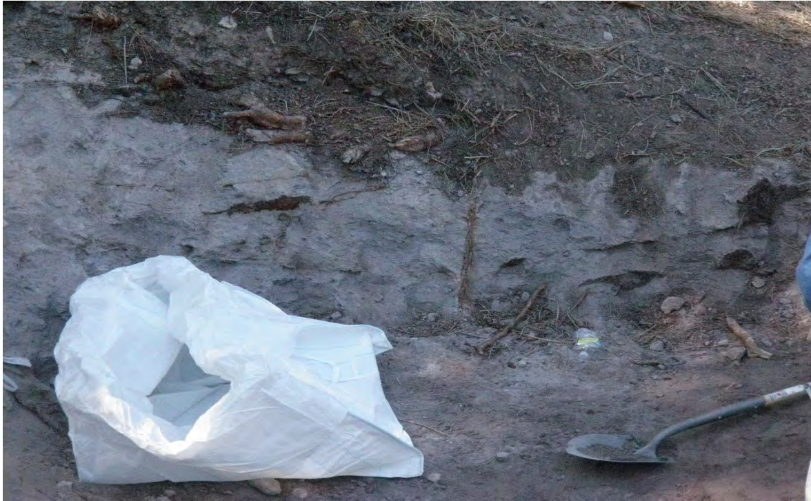
Shovel removal and packaging of contaminated media within the SWMU 01-001(f) outfall area
