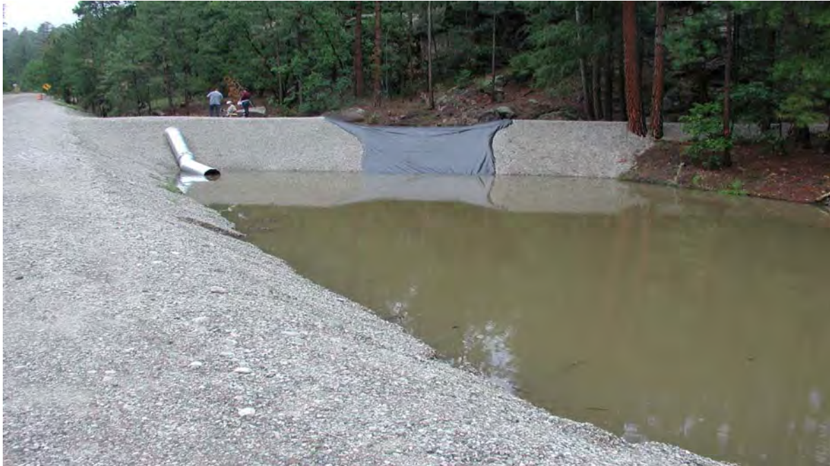
View of lower retention basin looking west on July 26, 2010, following three days of rain
