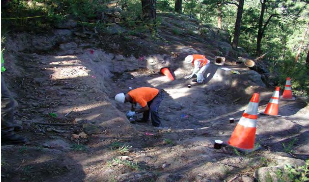
Collection of confirmation samples at Excavation Area 1 within the SWMU 01-001(f) outfall
