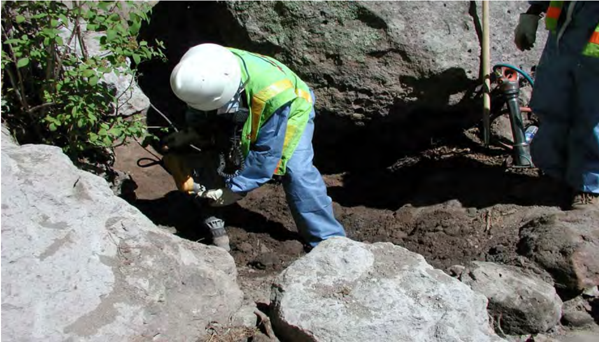
Removal of contaminated media from the drainage below the SWMU 01-001(f) outfall
