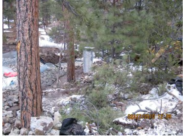
Photo 2 Gage Station stilling well, looking northeast from access road
