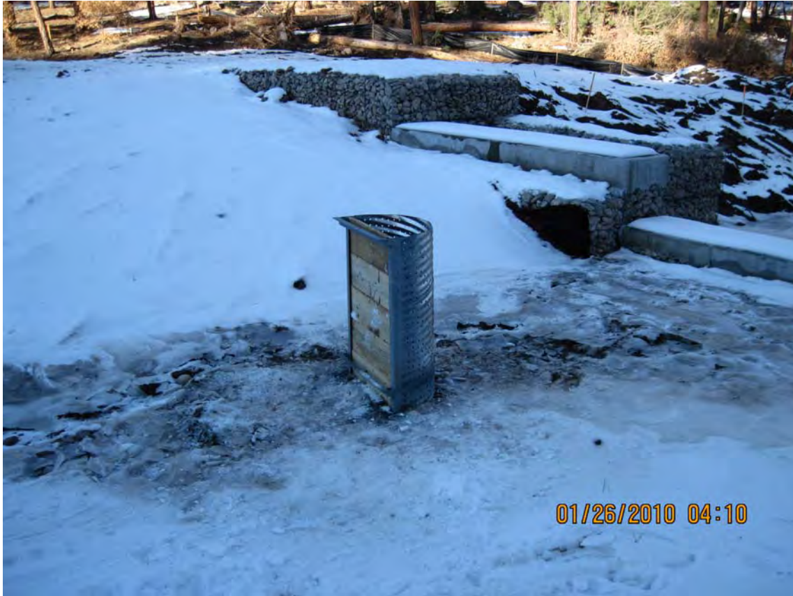
Figure 2.1-4 Adjustable riser pipe extended in height to match overflow weir crest height, low-flow and overflow weirs in background
