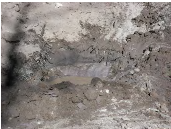
Photo 9 Stilling basin water intrusion
