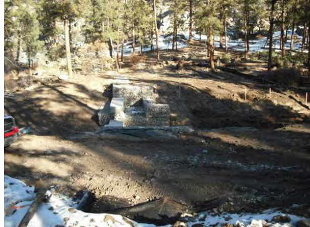
Photo 2 Structure, looking north, downstream north slope prepared for Class B rip rap installation
