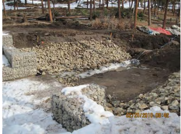
Photo 2 Class B rip rap on north slope, downgradient side of structure; pumping water from rip rap excavation area to keep flume subgrade dry
