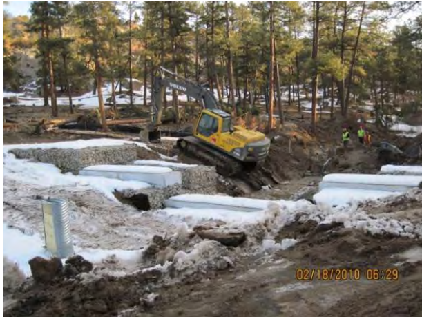
Photo 3 Downstream side of structure rip rap installation work, fully extended riser pipe in foreground
