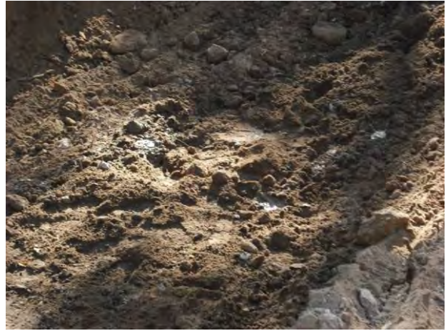
Photo 6 Water intrusion in north-half excavation
