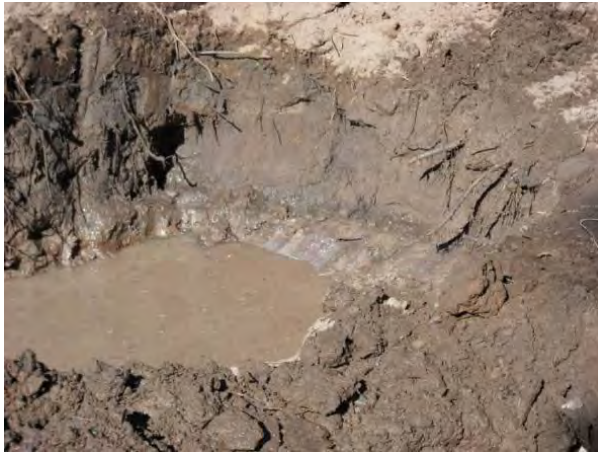
Photo 7 Water intrusion, high water mark in stilling basin excavation
