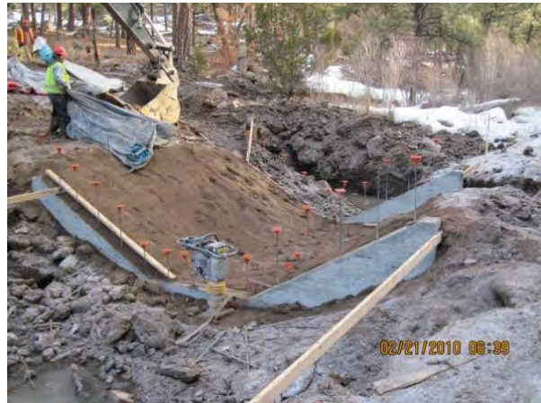
Photo 2 Removal of blanket from flume subgrade to continue preparation of flume subgrade
