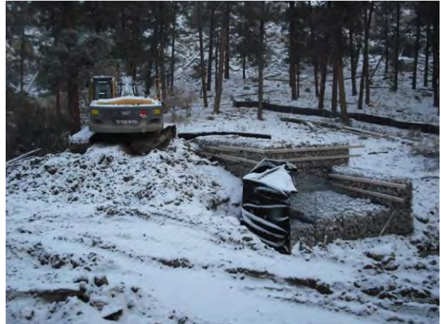
Photo 4 Structure with geotextile fabric wrapped on upstream face on north half of structure
