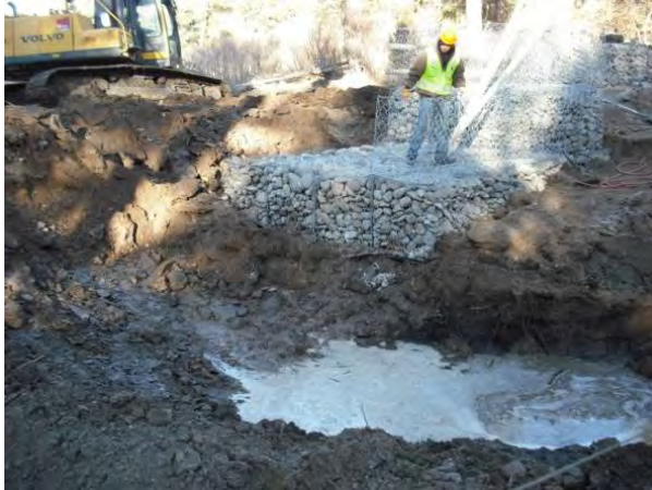
Photo 5 North-half structure construction; water intrusion in stilling basin excavation
