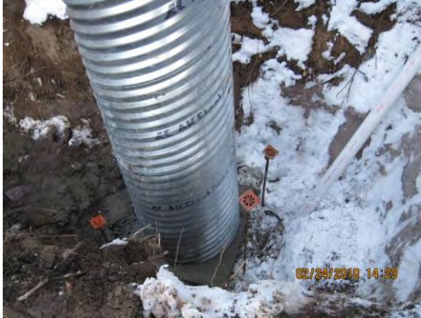
Photo 13 Gage Station stilling well placed in concrete
