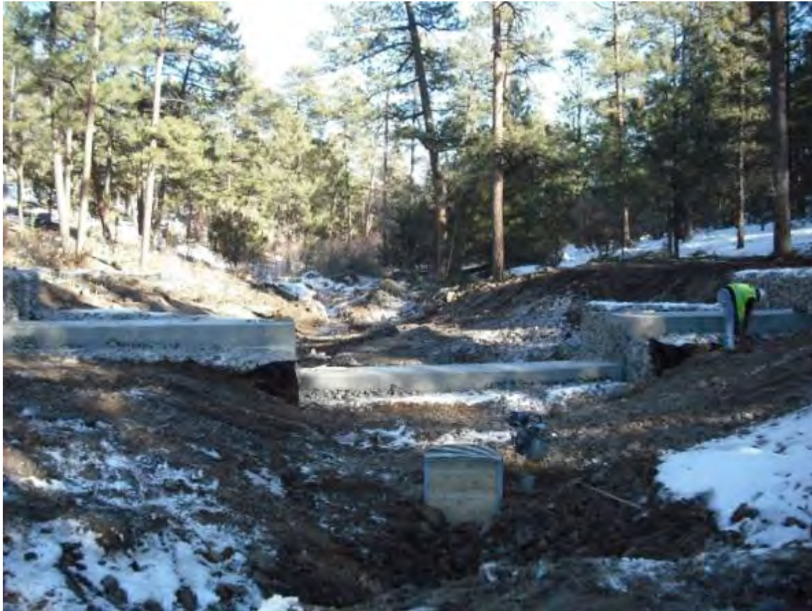
Figure 2.1-2 DP grade-control structure (looking east), low-flow and overflow weirs shown (riser pipe in foreground)
