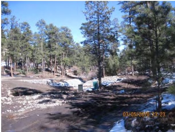
Photo 3 Looking downstream at structure, riser pipe in foreground and flume in background
