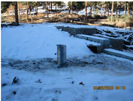
Photo 1 Riser pipe (fully extended) looking northeast
