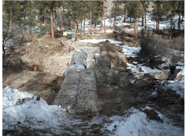
Photo 4 Concrete cap covered for curing, structure facing north, water intrusion downstream of stilling basin
