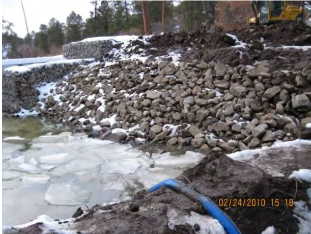
Photo 15 Photo of water being pumped from upstream of flume to keep flume area dry
