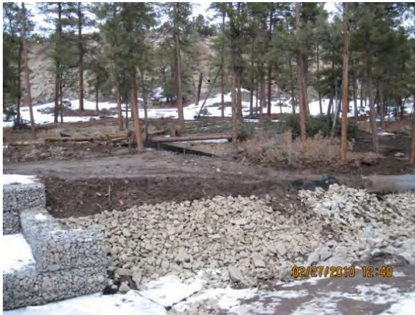
Photo 3 Completed Class B rip rap on north slope, on downgradient side of structure
