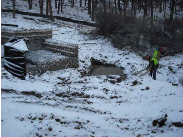
Photo 3 Structure with geotextile fabric wrapped on upstream face, on north half of structure, pumping groundwater from stilling basin excavation
