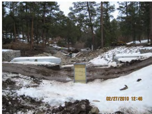
Photo 6 Upstream face of structure; riser pipe in foreground and flume in background
