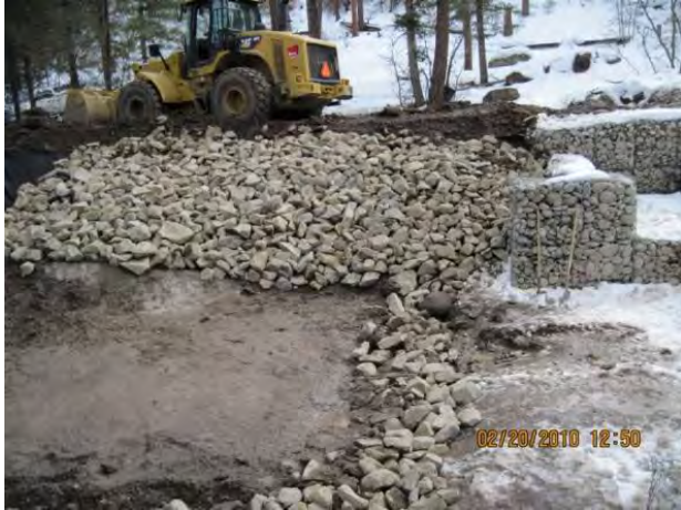
Photo 5 Class B rip rap, on south slope and downgradient of stilling basin, looking south
