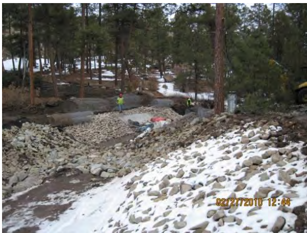
Photo 5 Completed Class B rip rap, upgradient of flume; Class A rip rap installation continues
