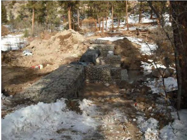
Photo 3 Concrete cap covered for curing, structure facing north, water intrusion downstream of stilling basin
