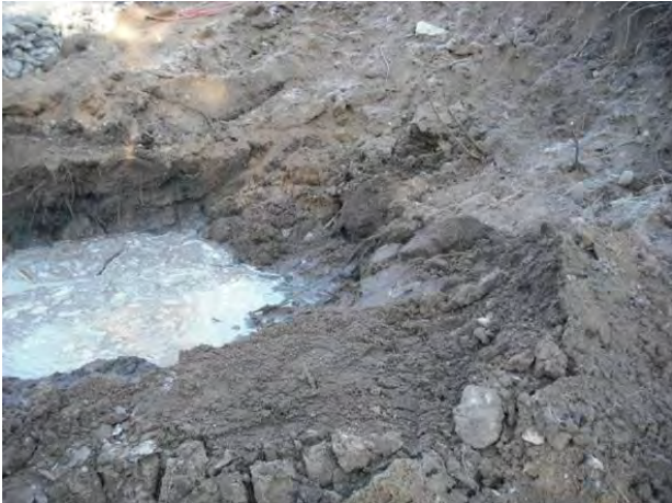
Photo 3 Water intrusion in stilling basin excavation
