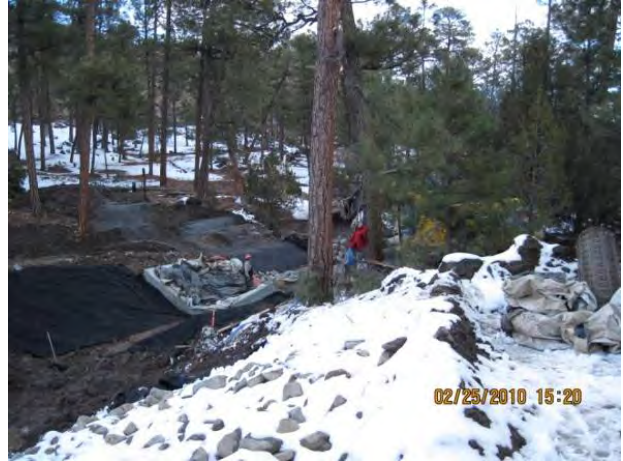
Photo 2 Flume concrete covered with concrete blankets to cure, looking northeast from access road
