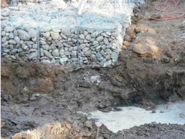
Photo 1 Water intrusion in stilling basin excavation
