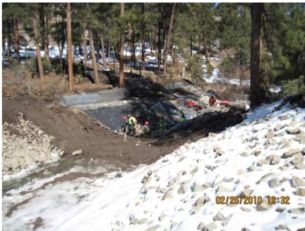
Photo 1 Installation of Class A rip rap on upstream and downstream sides of flume
