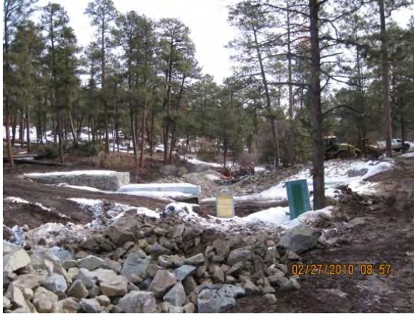
Photo 1 Upstream face of structure with downstream rip rap and flume in background
