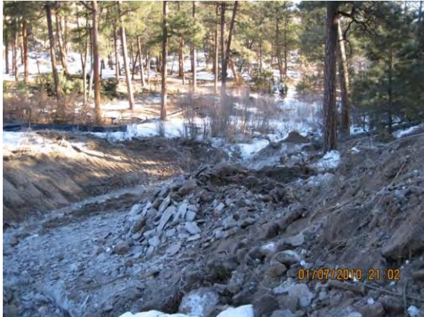
Photo 3 Excavation for downstream installation of Class A and Class B rip rap
