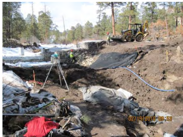
Photo 2 Class B rip rap installation, on north slope, downgradient of structure; water being pumped from Class B excavation area
