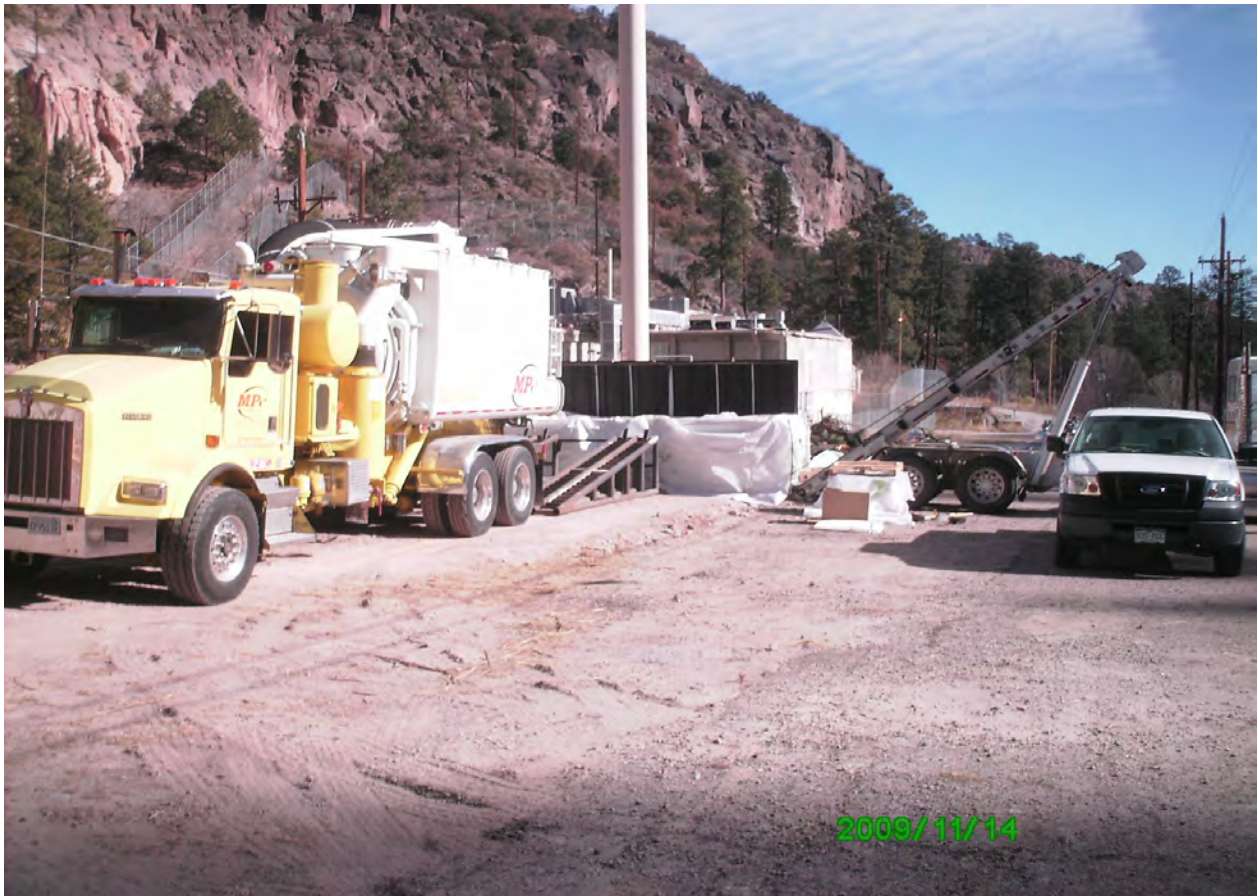
Vacuum truck and rolloff bin
