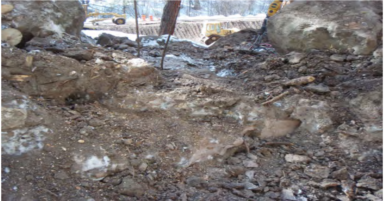
Bottom of drainage and construction of new retention pond in canyon bottom below
