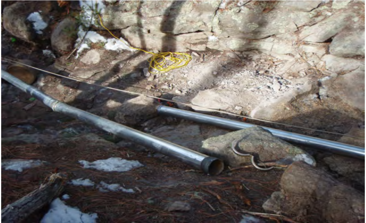
Vacuum pipe within drainage
