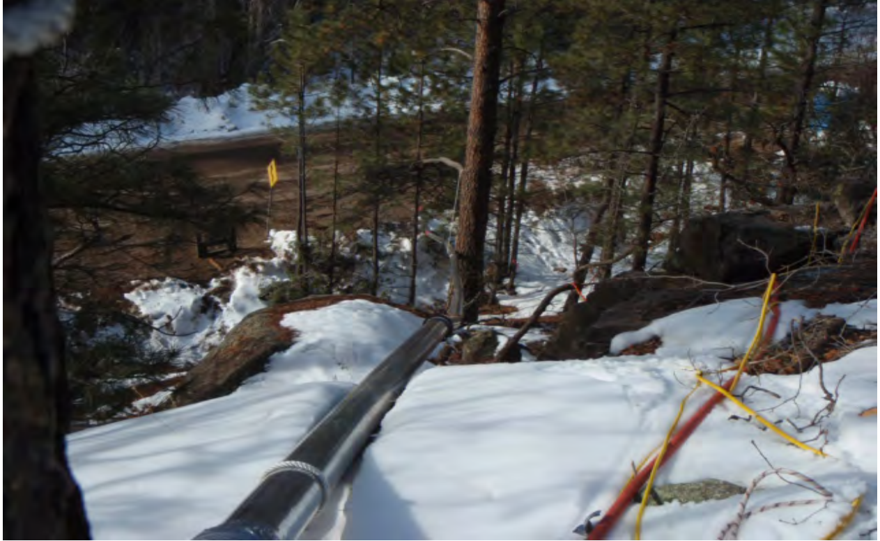
View of vacuum pipe at bottom of drainage and canyon bottom
