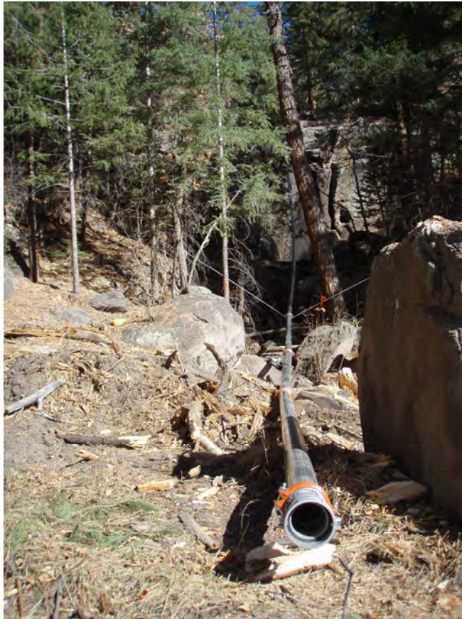
November 2009, vacuum pipe installed updrainage
