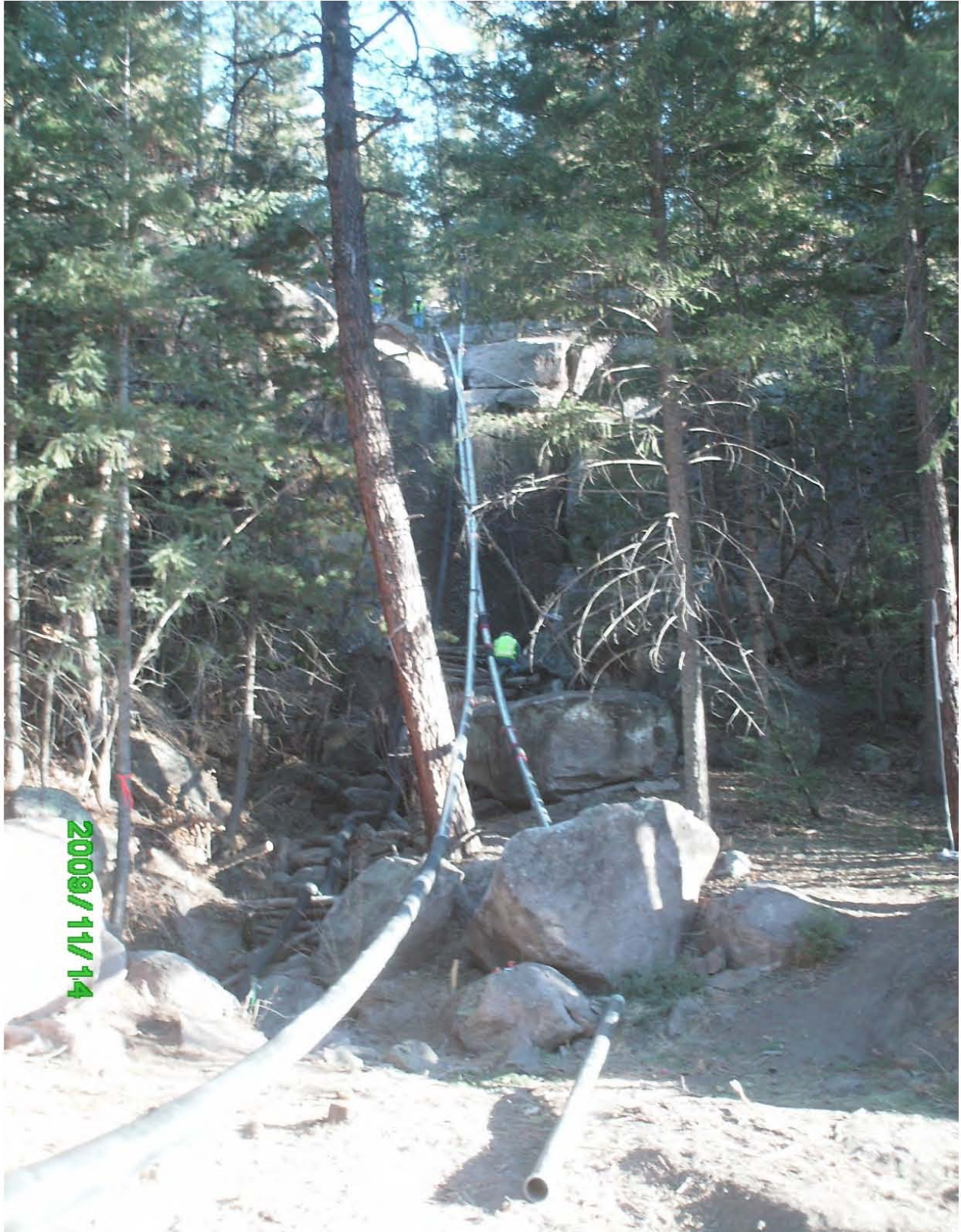
View of vacuum piping from bottom of drainage
