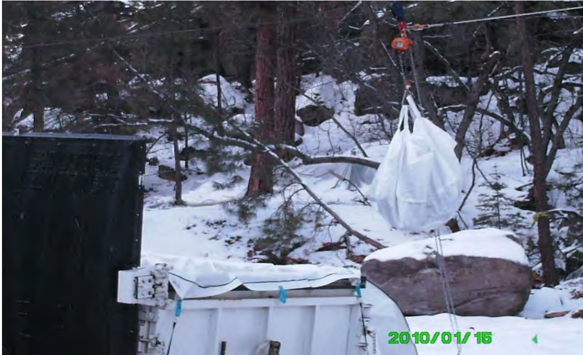
Bags of excavated rock from drainage transported on slip line to rolloff bin
