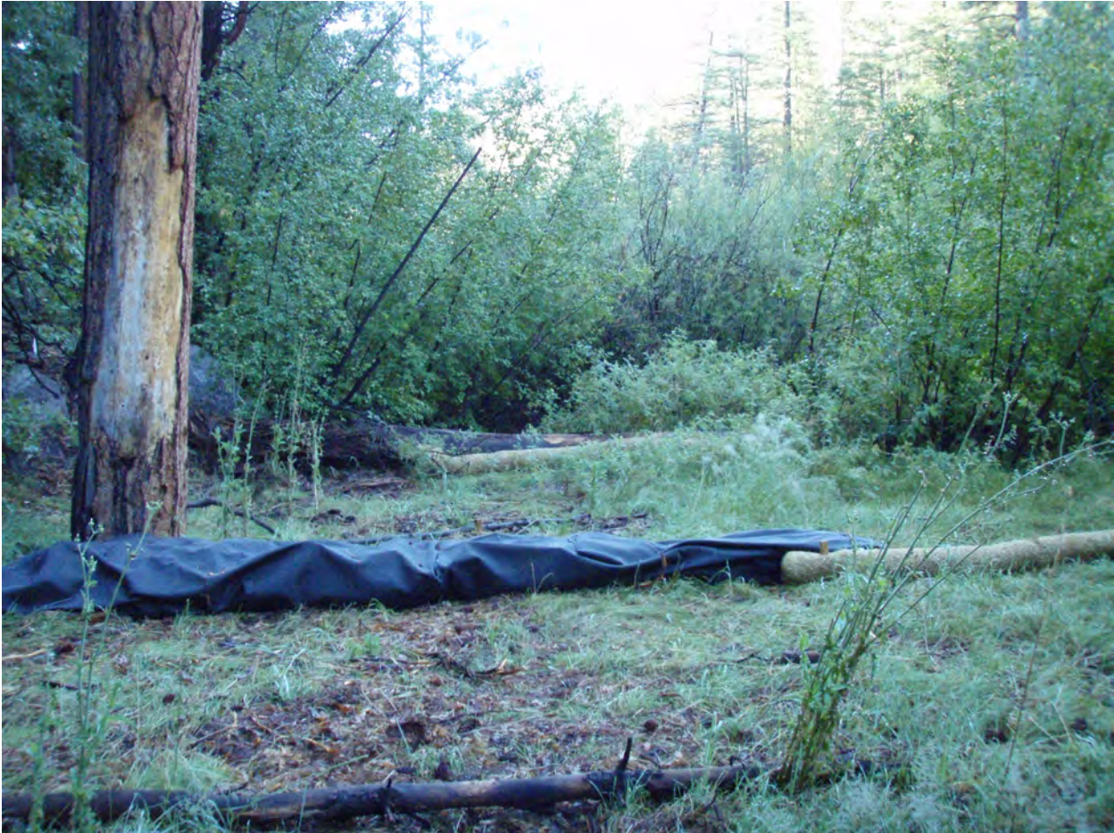
July 2009, looking east at filter wrapped juniper bales and wattles. Placed in historical channel and flood plain to enhance infiltration and sediment retention.
