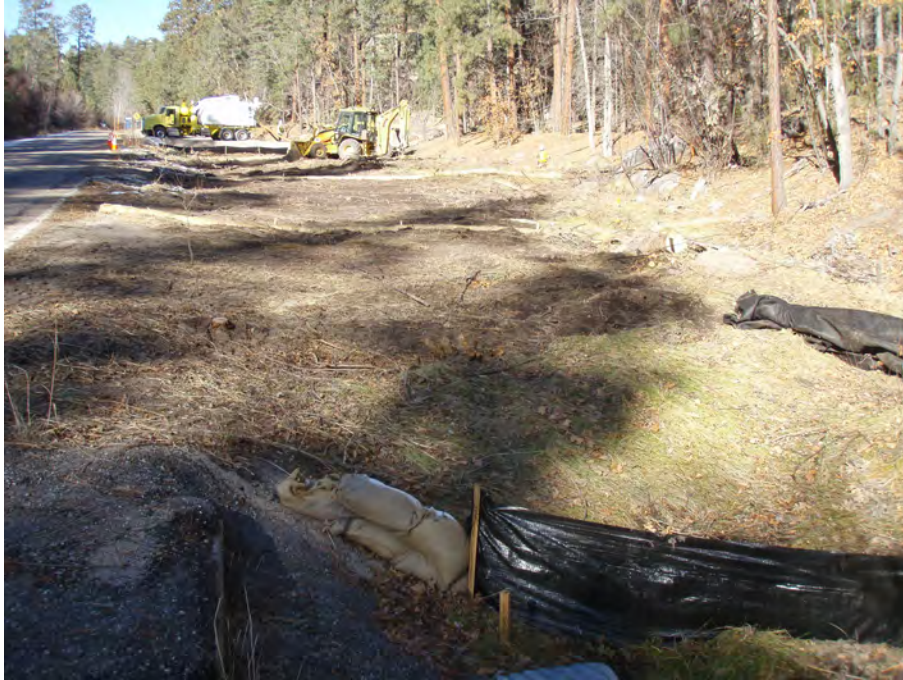
November 2009 looking upcanyon. Trees and brush have been removed from proposed pond area and temporary best management practiccess installed. Vacuum truck on pad.
