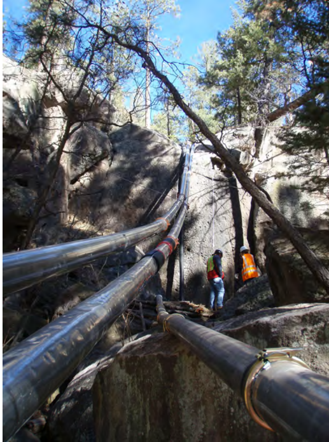
November 2009, multiple piping runs updrainage to facilitate the use of two vacuum trucks
