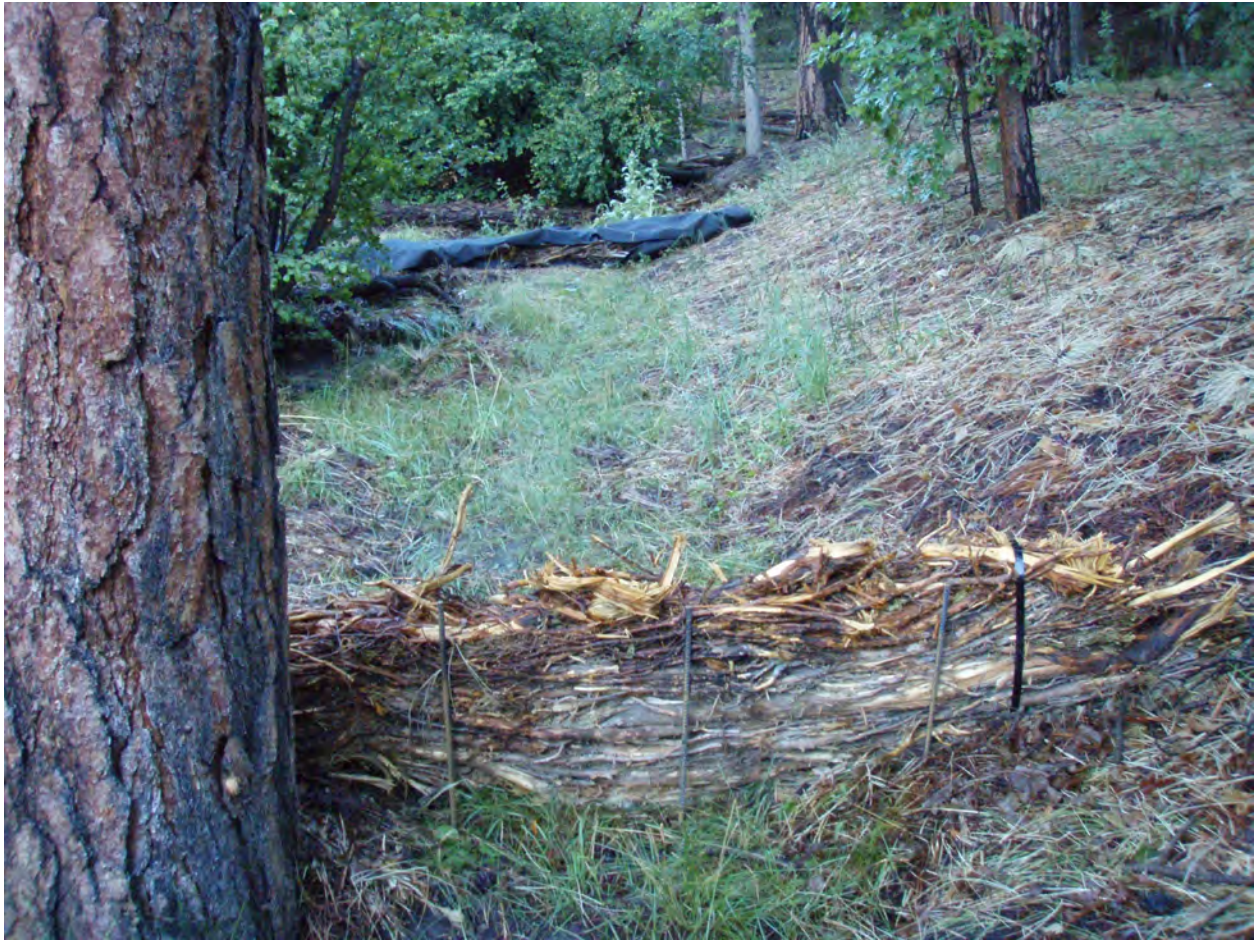
July 2009, looking west at juniper bales (wrapped in filter fabric and open). Bales placed in historical channel to enhance infiltration and sediment retention.
