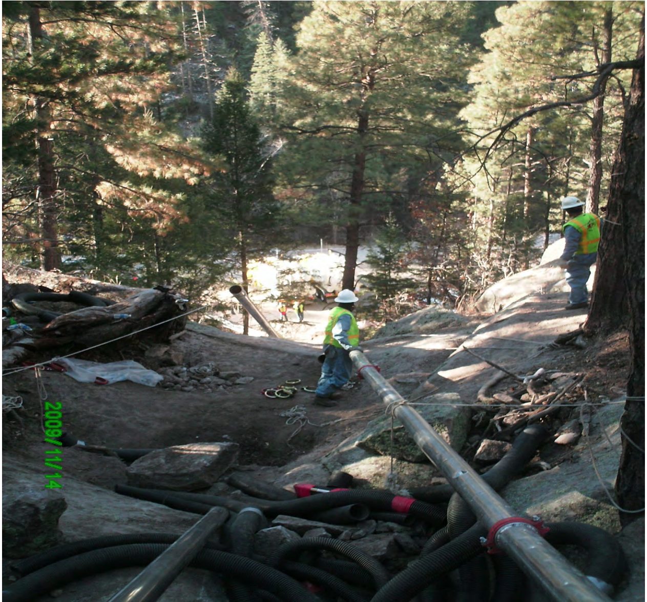
View of crews setting up vacuum piping from drainage looking toward canyon bottom
