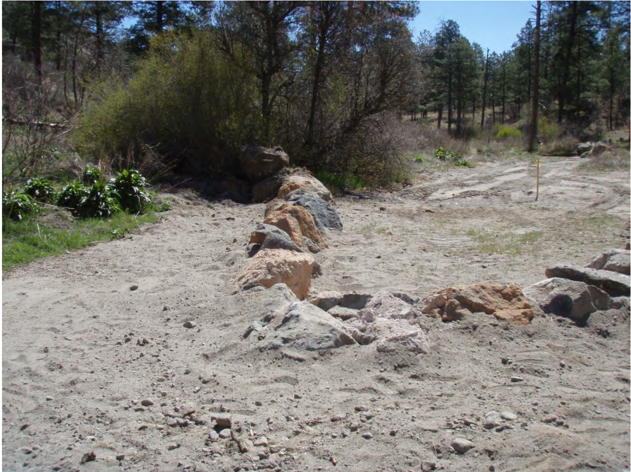
Figure 1 Pueblo Canyon cross vane 1 looking eastward (downcanyon). Note that the vertex of the structure is at stream-bed elevation.
