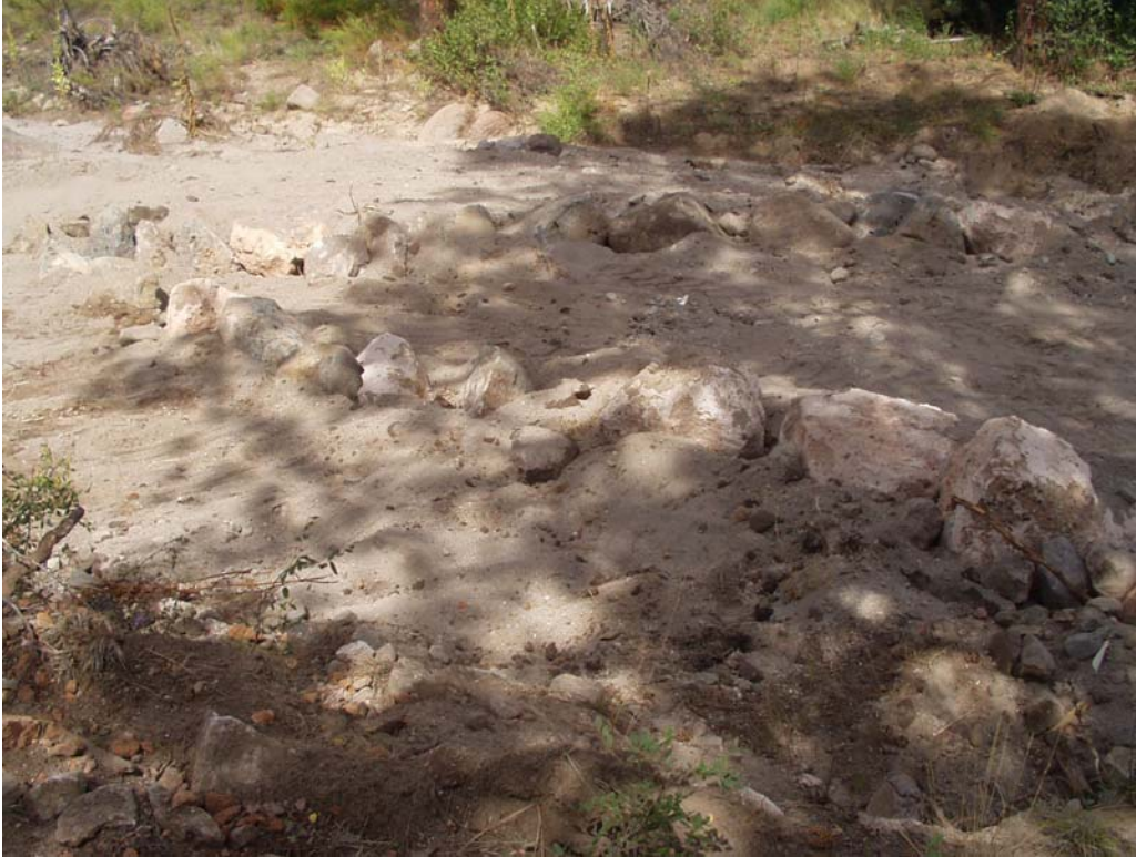
Figure 1a View of upper cross-vane structure looking north across the Pueblo Canyon channel
