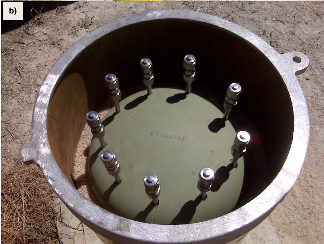
a) Nine port vapor-monitoring well installed at BH 21-25262 b) Nine port vapor-monitoring well head completion for BH 21-25262
