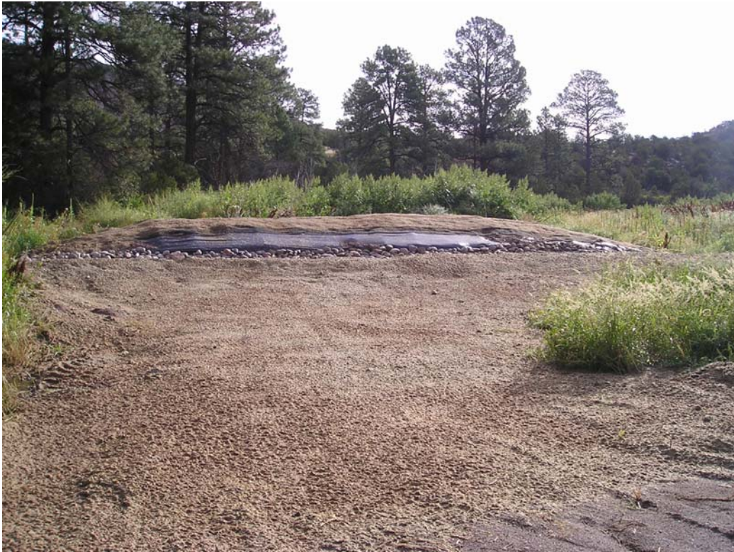
Figure 5 View looking down Pueblo Canyon. Stabilized wing ditch berm and rock liner are visible. Hydromulched surface is visible in foreground. Main Pueblo Canyon channel is just to the left of area shown in the photo.
