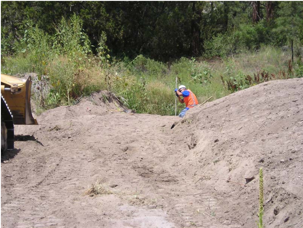
Figure 2 View looking upgradient along wing ditch towards existing channel. Initial excavation and surveying for grade.
