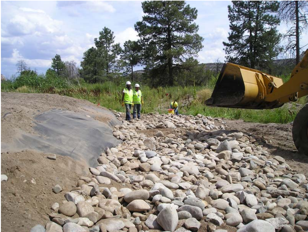
Figure 3 View looking downgradient along wing ditch. Placement of geotextile and rock liner.
