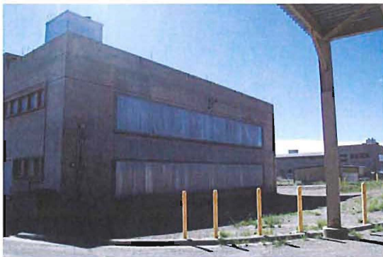
West side of Wing 4. Note blow-out panels and glass block panels on the north side (left)
