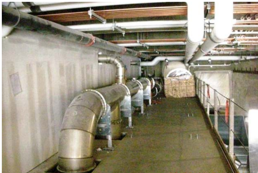
Laboratory level duct work
