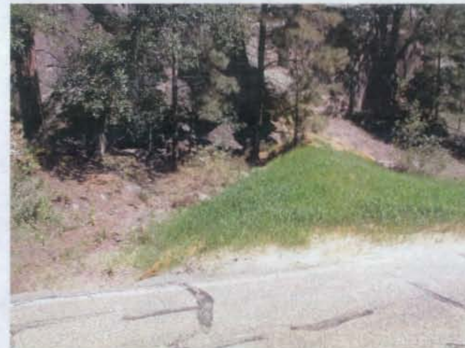
Figure 3.1-2 Earthen berm that routes stormwater under paved road through 18-in. culvert and away from LA-SMA-2 drainage
