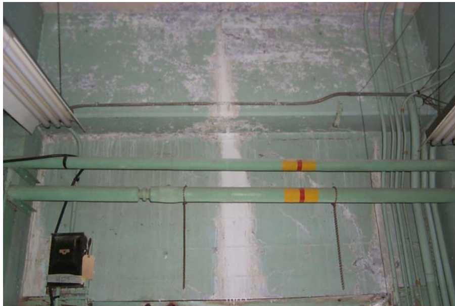
Figure 12. TA-8-1 interior water damage
