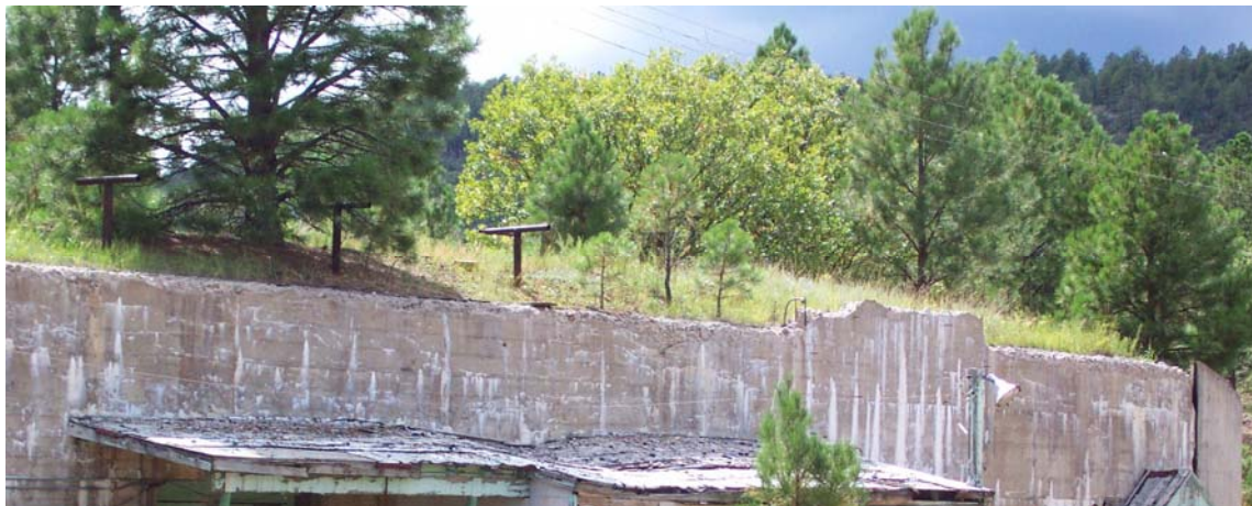
Figure 13a. TA-8-1, concrete spalling at parapet, looking southwest
