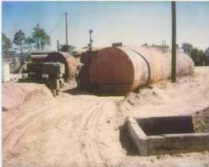
TA-3-17B Asphalt Oil Storage Tanks (EMPTY) 85100 oil in 1, Emulsion in #2 V=N
