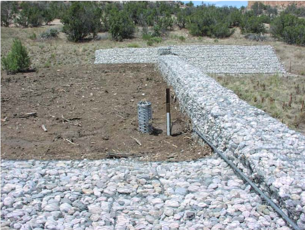
Figure 3.4-3 Photographs of Los Alamos Canyon low-head weir and upstream sediment retention basin on March 30, 2001 (top; view to the west) and July 10, 2006 (bottom; view to the north)
