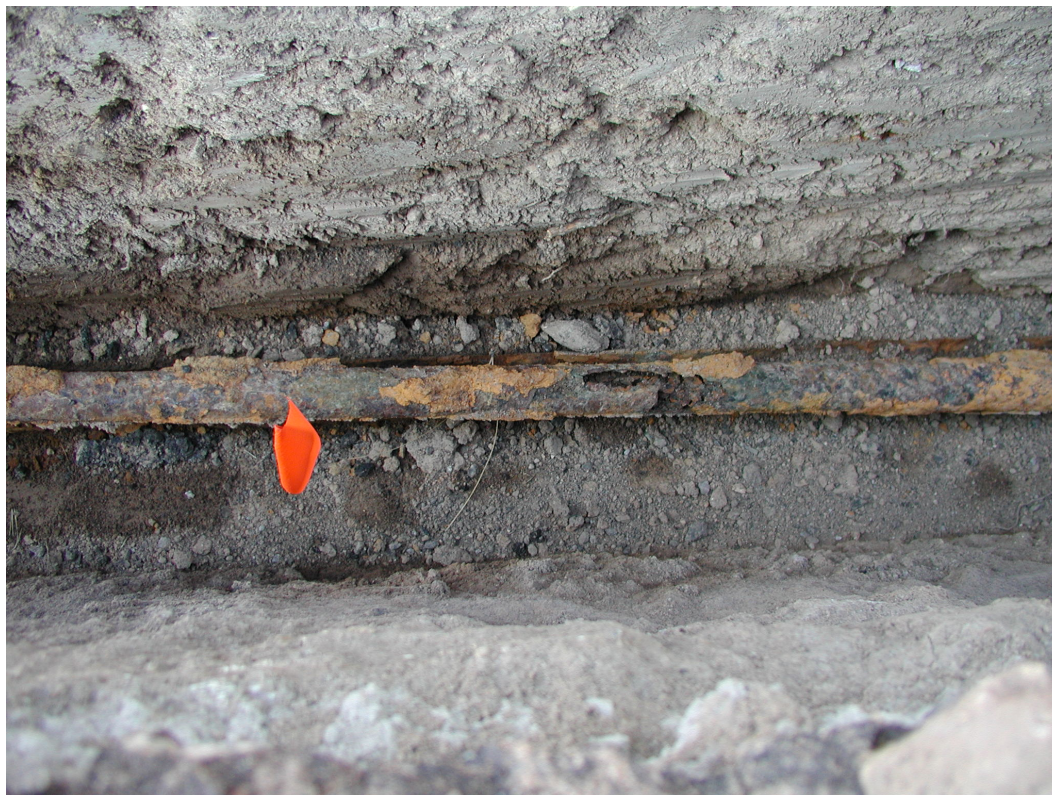
Figure B-9 Once exposed, numerous holes were visible in the steel drainline.
