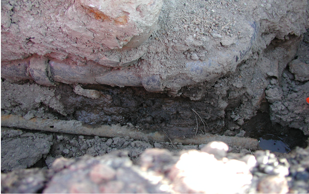
Figure B-15 A damaged portion of the roof drainline at the second elbow. This section was later repaired by splicing in a section of PVC pipe. The steel drainline is also visible and has been cut before removal.
