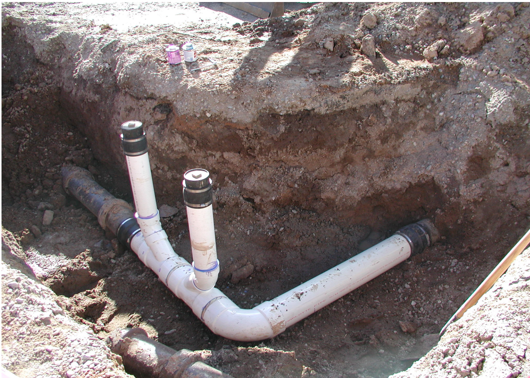
Figure B-16 Before backfilling, the second elbow of the roof drainline was repaired by splicing in a section of 6-in. PVC.
