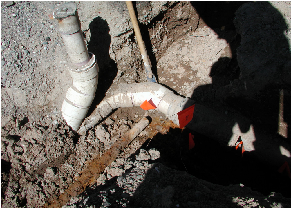
Figure B-14 Polyvinyl chloride (PVC) pipe was used in a recent repair of the roof drain at the first elbow. The steel drainline has been cut and is ready to be removed from the trench.
