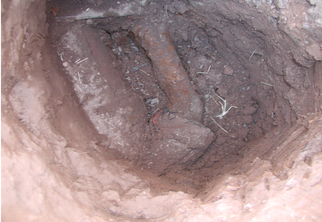
Figure B-17 The location where the 2-in. steel drainline connects to the 6-in. clay roof drainline
