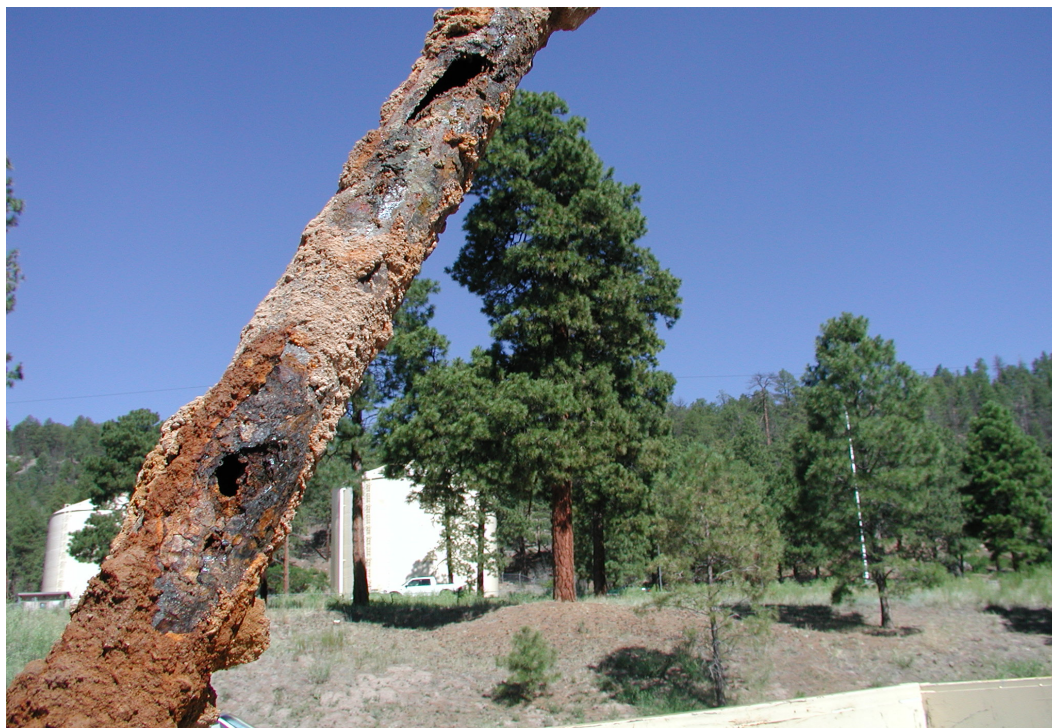
Figure B-10 The corroded drainline
