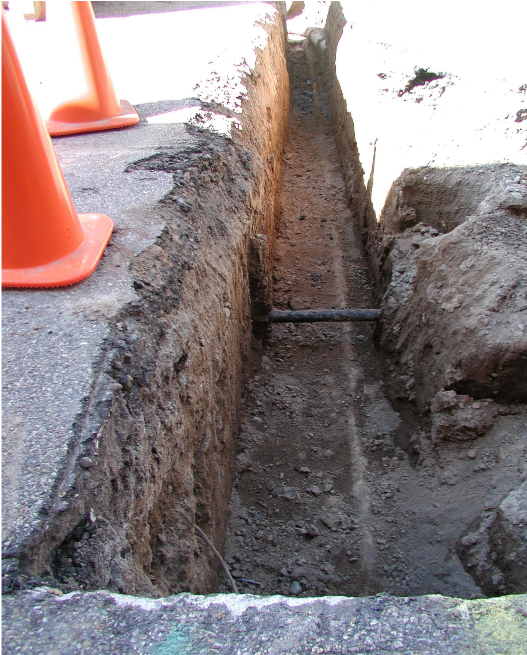
Figure B-8 Trench exposing the steel overflow line. A gas line crosses the trench and the 6-in. roof drainline is visible near the top of the photograph.
