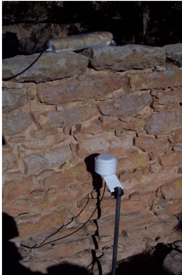
Figure 12. Displacement and temperature sensors.
