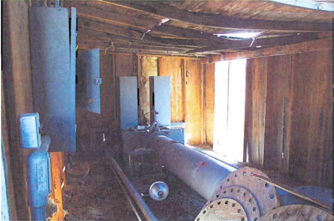
TA-49-121, Hydraulic Ram Enclosure, direction southeast (2005)
