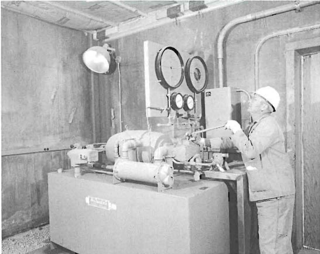
TA-49-23, hydraulic compressor for the Cable Test Facility (TA-49-121) (1971)
