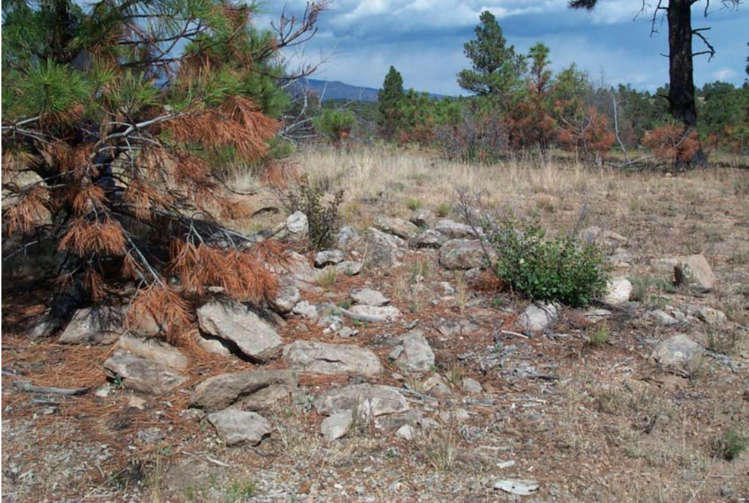
Figure 9.10. LA 89760, a one- to three-room structure with a partially burned tree that poses a threat to site masonry.
