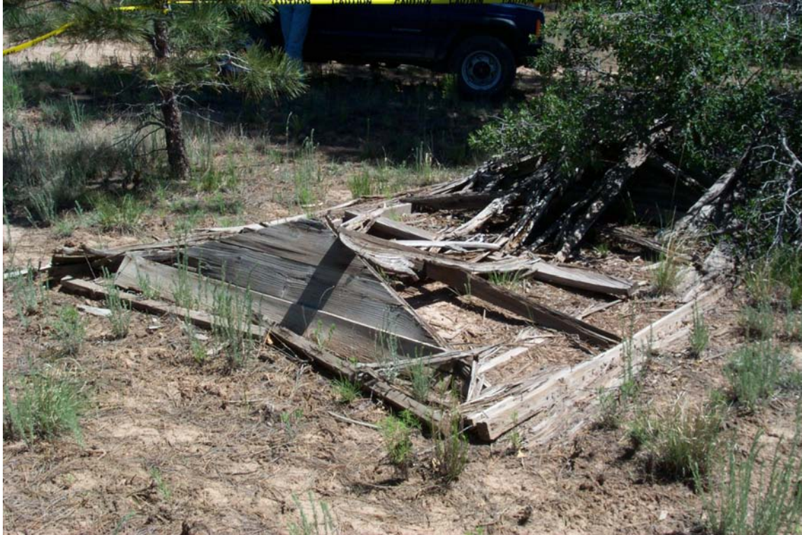
Figure 12.9. LA 131234, Structure C after the Cerro Grande Fire.
