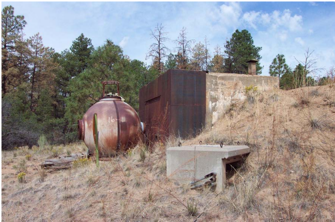
Figure 11.10. TA-14-5, rear view of former control room and berm after the Cerro Grande Fire.
