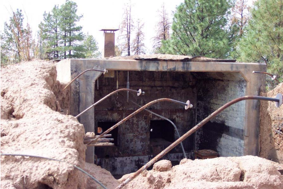
Figure 11.9. TA-14-5, remaining concrete portion and berm after the Cerro Grande Fire.
