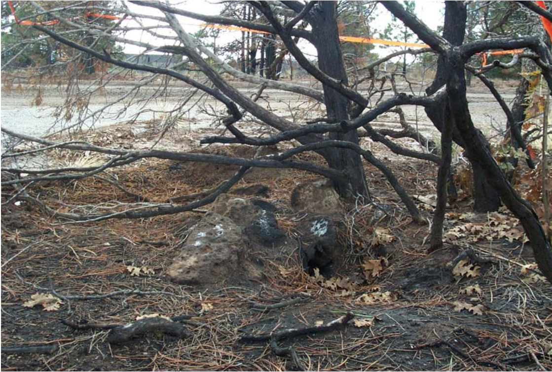
Figure 9.16. LA 136793, a one- to three-room structure impacted by fire and suppression activities; removal of snags and fencing of the site is recommended.
