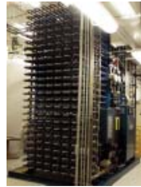
Tubular ultra-filter after major rebuilding, September 2001.
