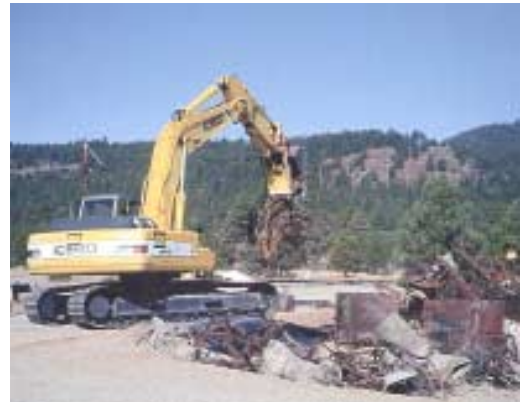
A remote operated excavator was used to uncover burning debris at TA-16 after the Cerro Grande fire
