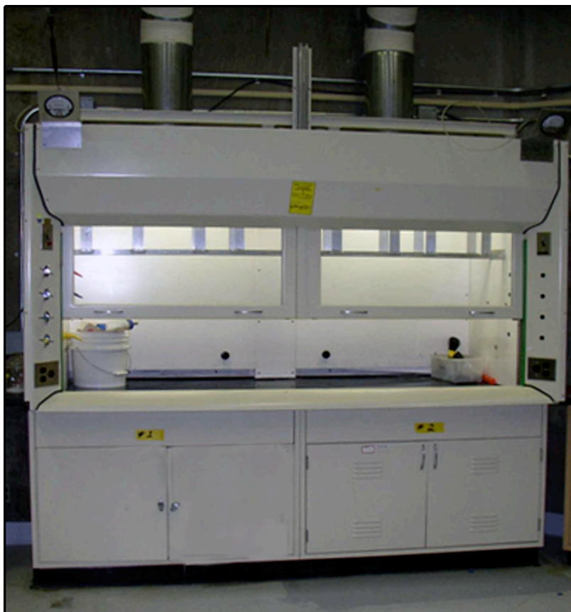
Figure 2.10-1 Example of chemical use in laboratory hood at LANL.
