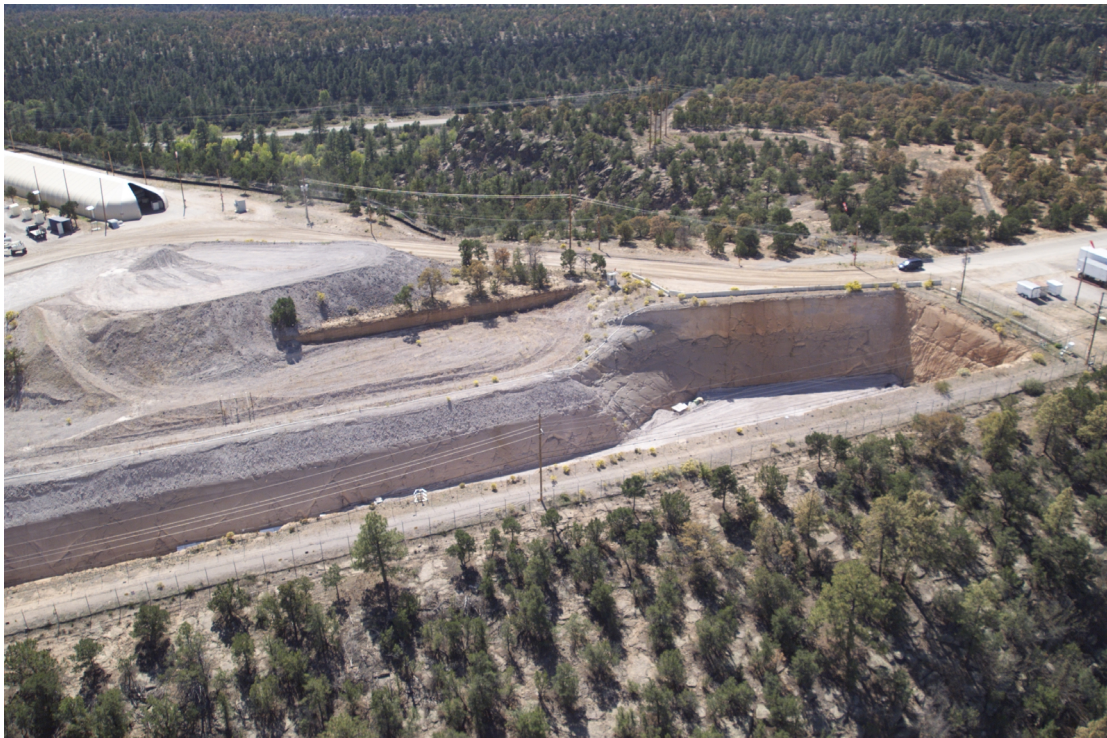
Figure 3. Aerial photo of the new waste trench at the northwest end of Area G.
