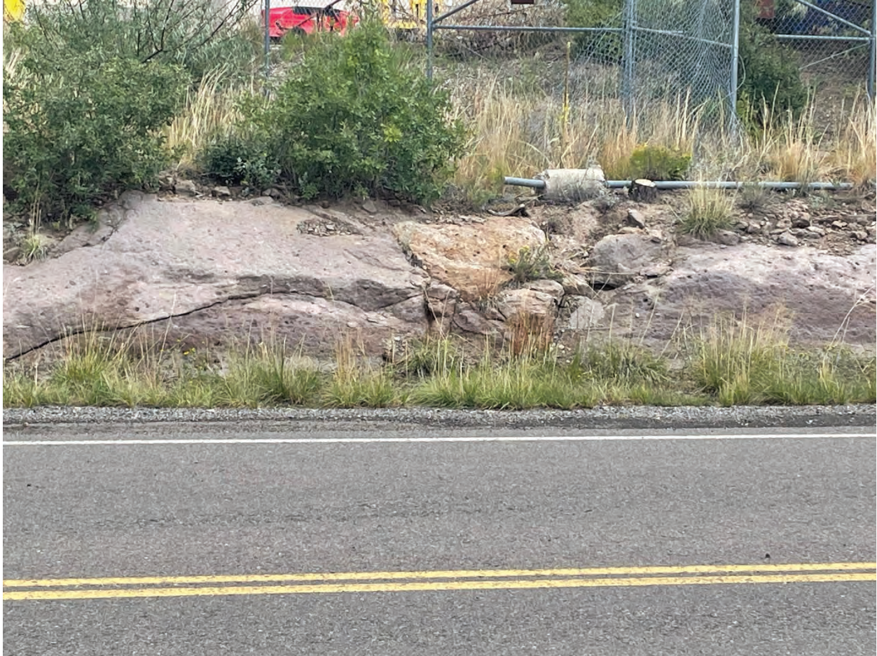
South of TA-60, Building 17, facing north at road cut on south side of fence
