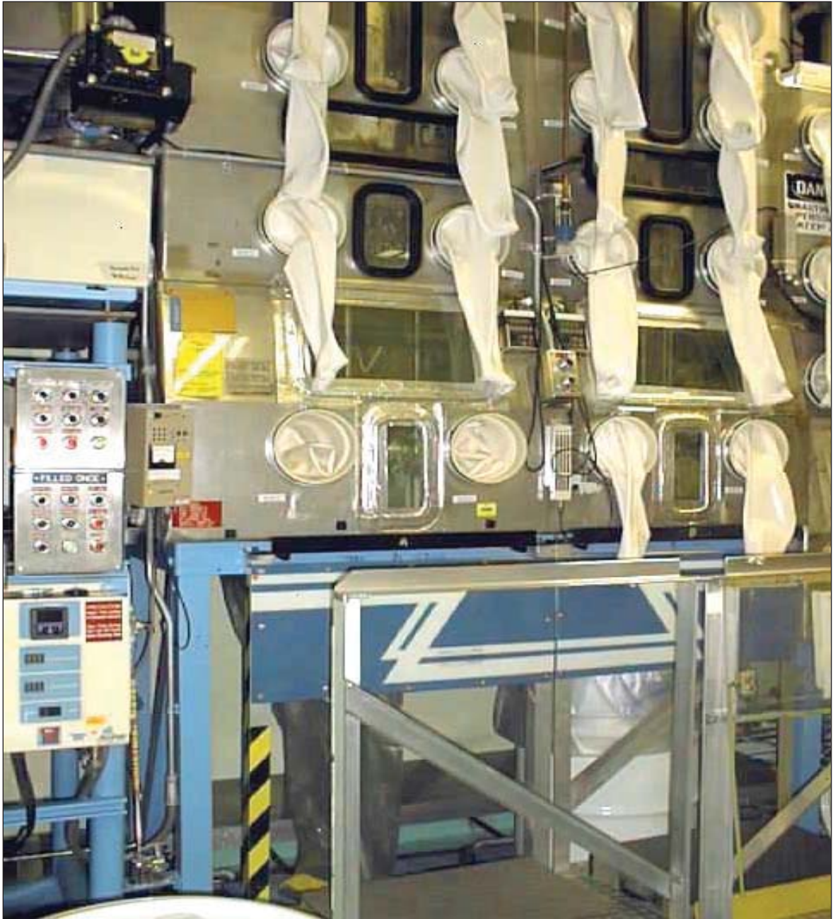
TA-55-4, Room 401, Stabilization Unit Process Code T04, Treatment Unit
