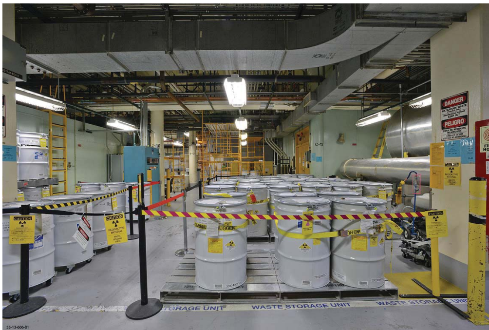
TA-55-4, Basement, Process Code S01, Container Storage Unit (B40) (View is looking southwest)
