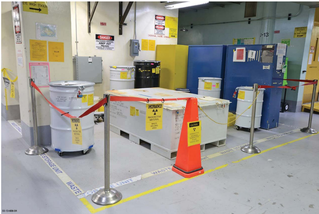
TA-55-4, Basement, Container Storage Unit K13, Process Code S01, Container Storage Unit
