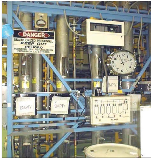
TA-55-4, Room 401, Stabilization Unit Pencil Tanks Component, Process Code S02, Storage Tank System
