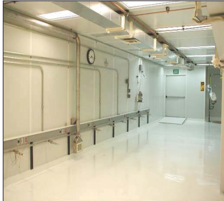
TA-3-29, Wing 9, Basement Room 9010, Process Code S01, Container Storage
