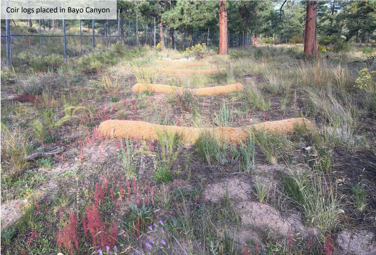
Earthen berm with TRM at the top of Pueblo Canyon
