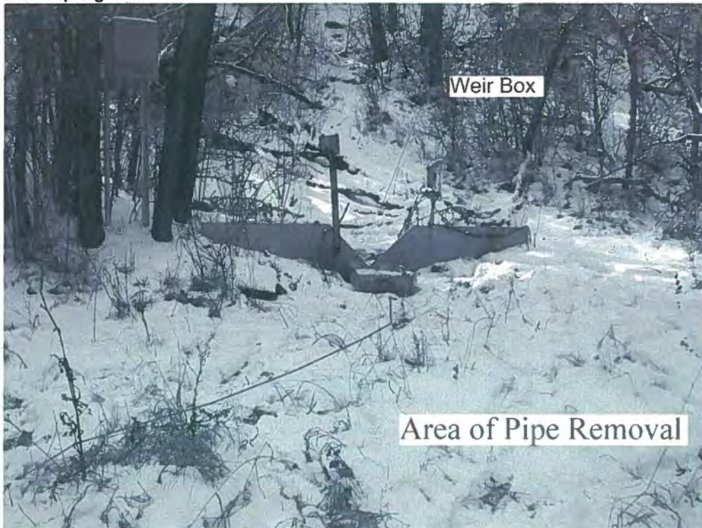
SWSC Spring Weir Box
