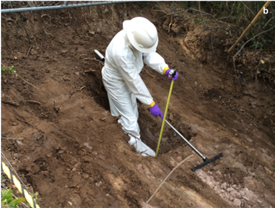
Photo A-4 Excavation activities within the cliff-top portion of SWMU 01-001(g) on U.S. Department of Energy property
