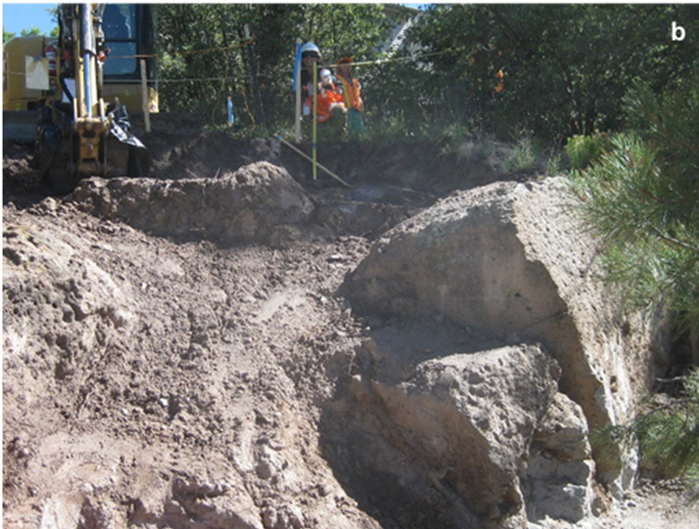
Photo A-3 Excavation of the “toe” or southern-most portion of the SWMU 01-001(g) outfall area
