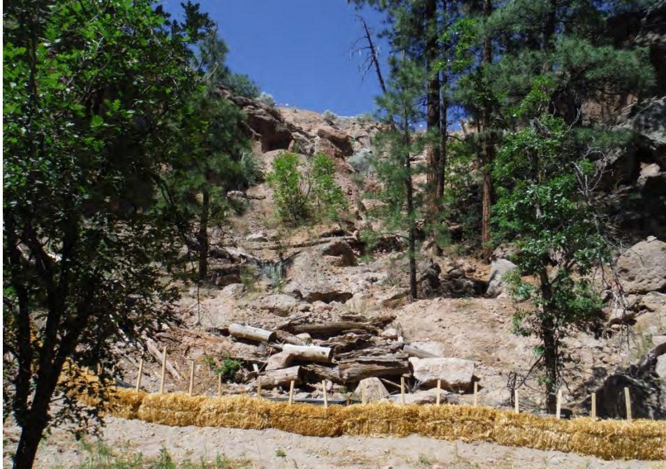
Figure E-2.2-4 June 2016: Newly installed best management practices above upper defense cell. Installation by Los Alamos County landfill operations.
