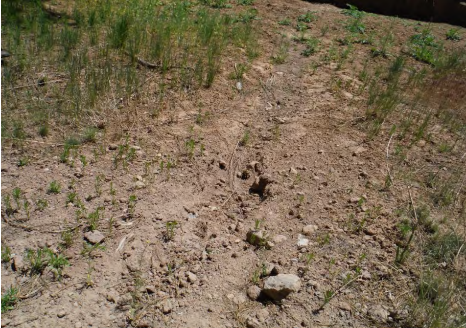
Figure E-2.2-2 June 2016: Minor rill showing in earth fill area between defense cells
