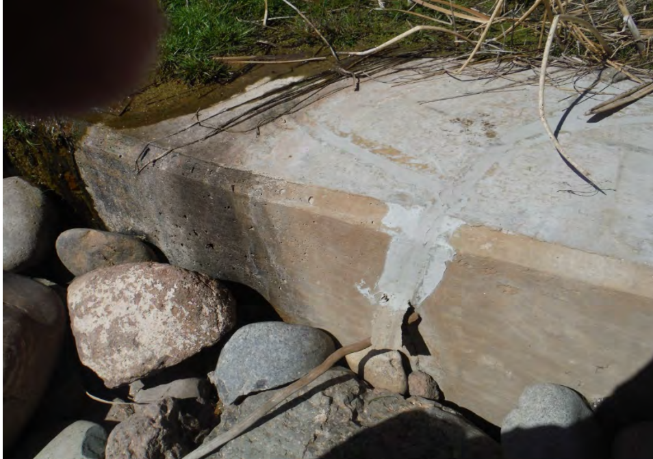
Figure E-2.4-2 March 2016: Previous crack repair on middle grade-control structure. No change from past inspections.
