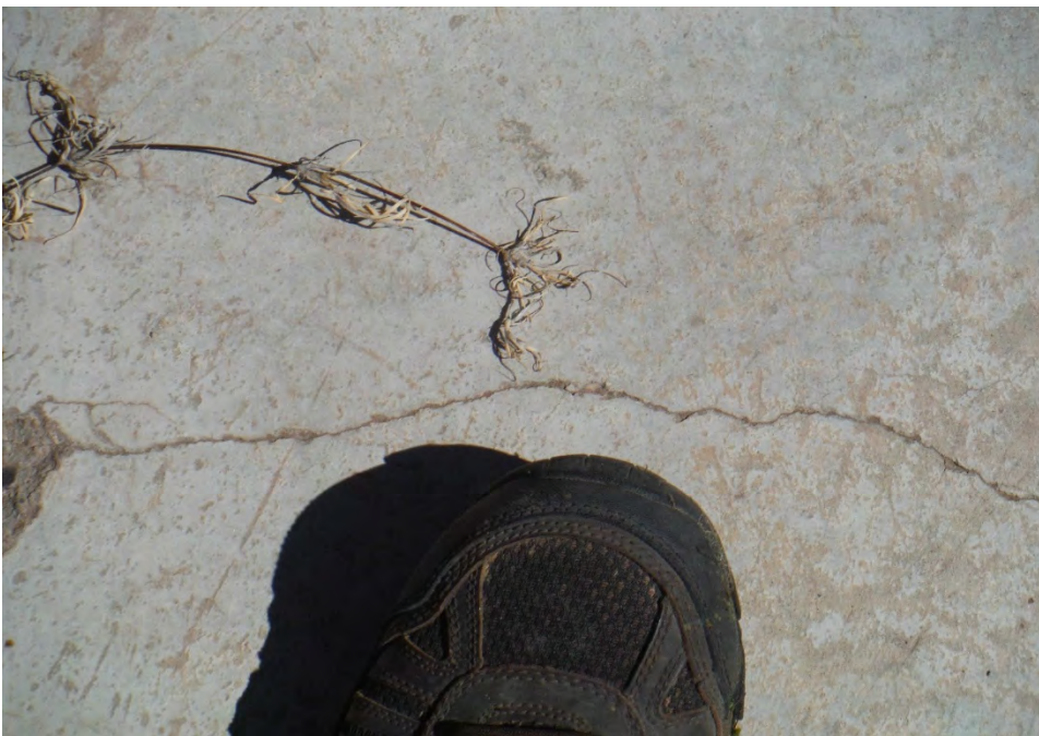
Figure E-2.4-5 March 2016: Crack monitoring. No change from last inspection.
