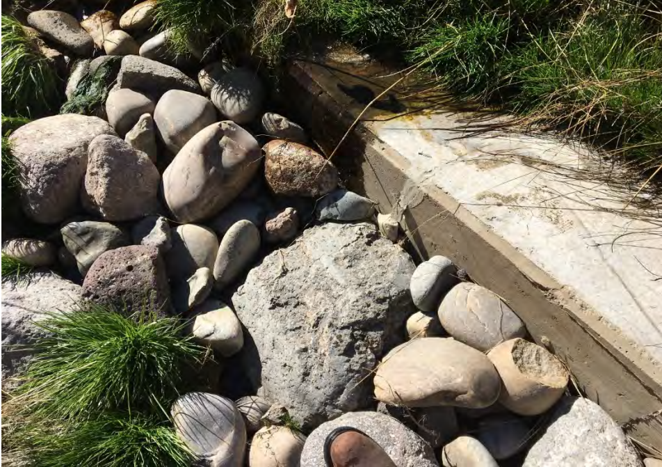
Figure E-2.4-4 November 2016: Crack repair on middle GCS. No change from past inspections.
