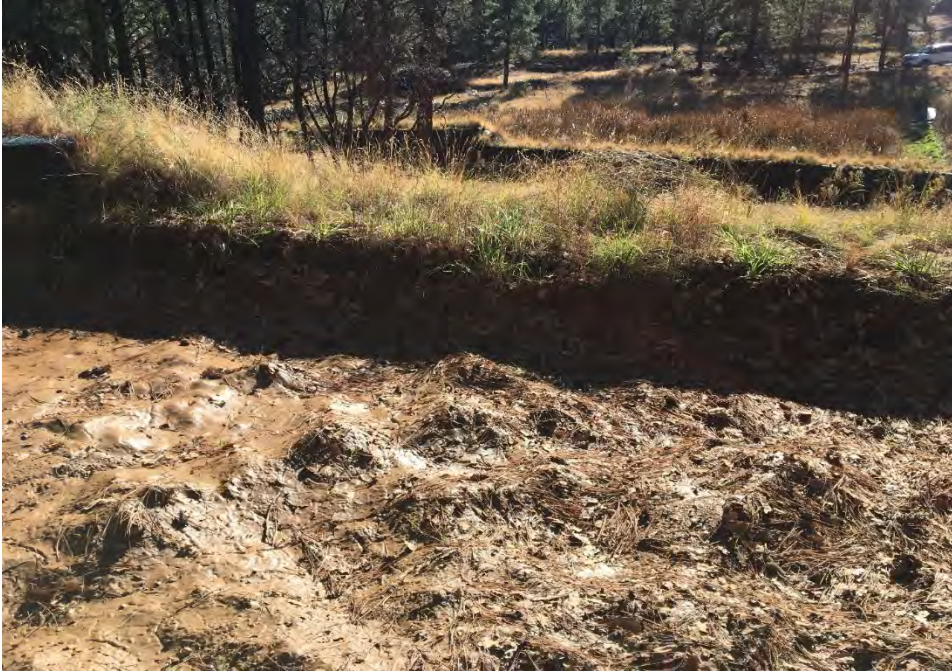
Figure E-2.2-6 November 2016: Upper defense cell muck intrusion from Los Alamos County landfill slope. Defense cell operating as designed.
