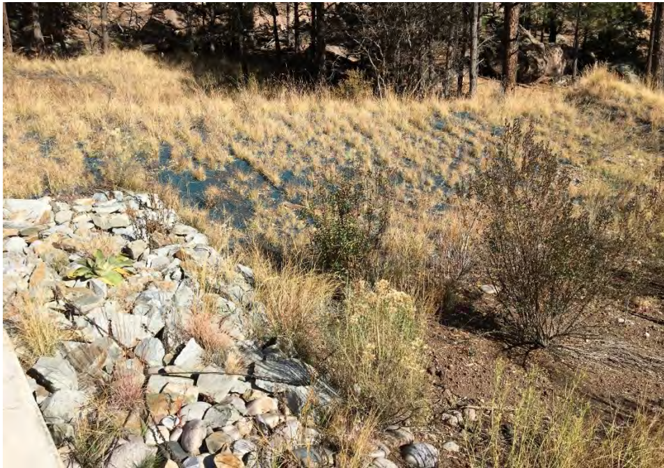
Figure E-2.1-6 November 2016: Vegetation on north embankment showing improving fill-in from March 2016 inspection
