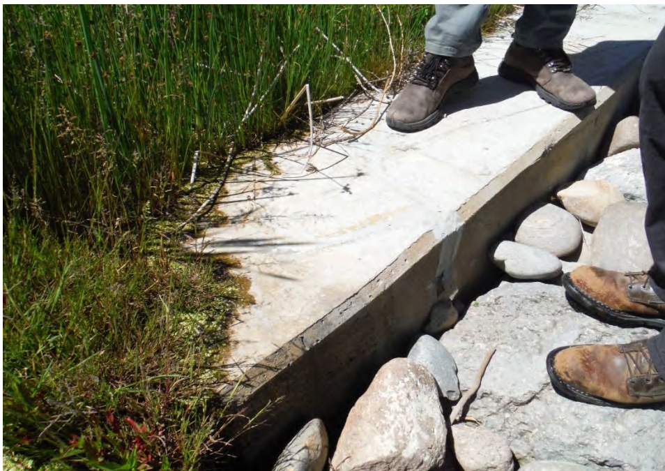
Figure E-2.4-3 June 2016: Crack repair on middle GCS. No change from past inspections.
