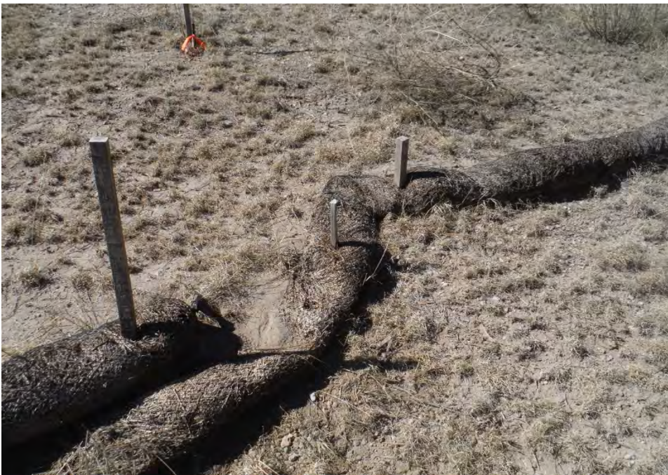
Figure E-2.4-1 March 2016: Straw wattle damaged by animal or persons walking on wattle. Recommend maintenance action.
