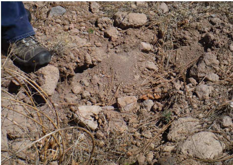
Figure E-2.2-1 March 2016: Earthen fill between upper and lower defense cells showing minor knick point (shifting material may lead to rill and erosional features)
