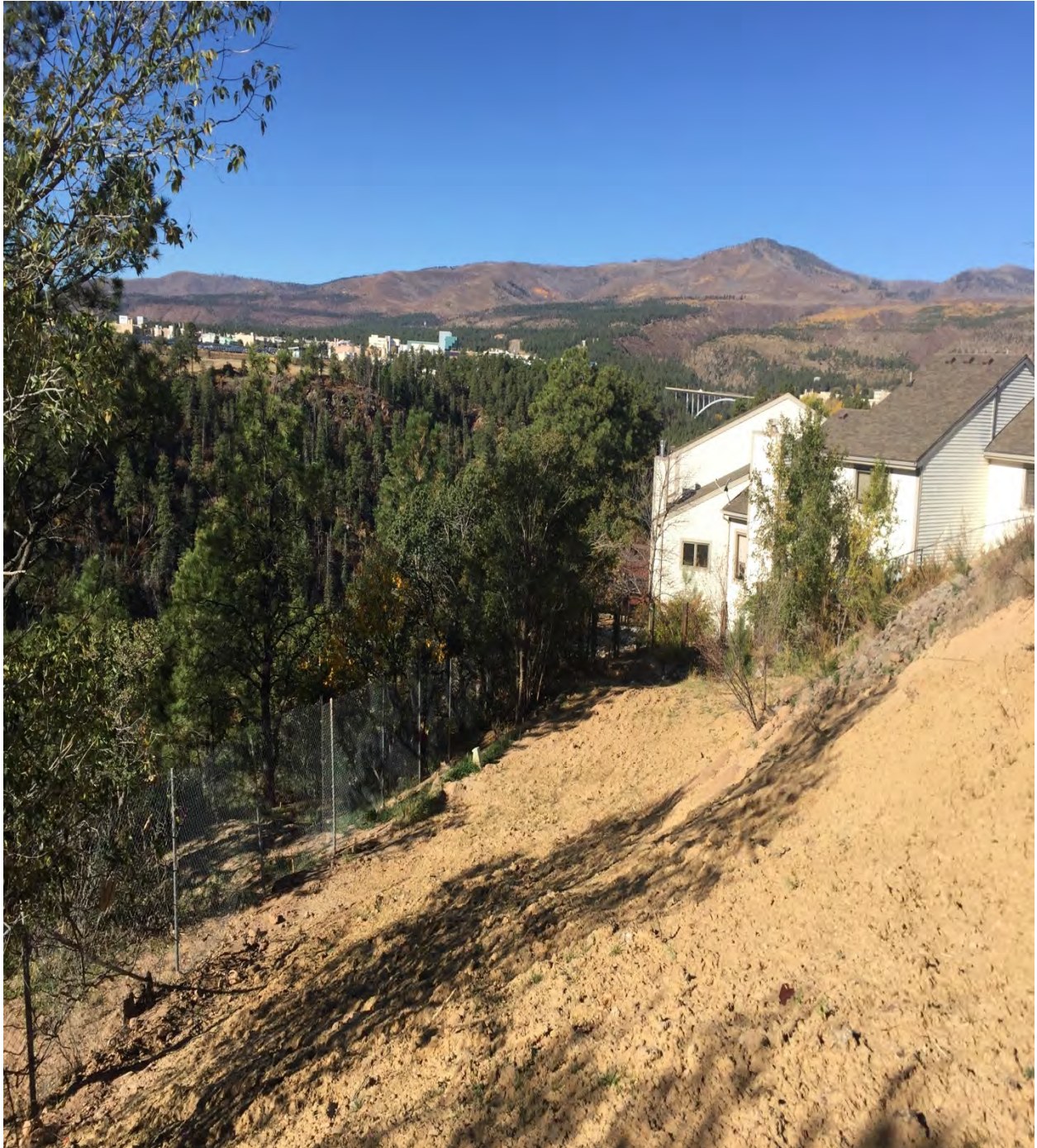
Figure H-6 SWMU 01-007(a) containing the former outfall area of SWMU 01-006(b) following recent remediation and site-restoration activities
