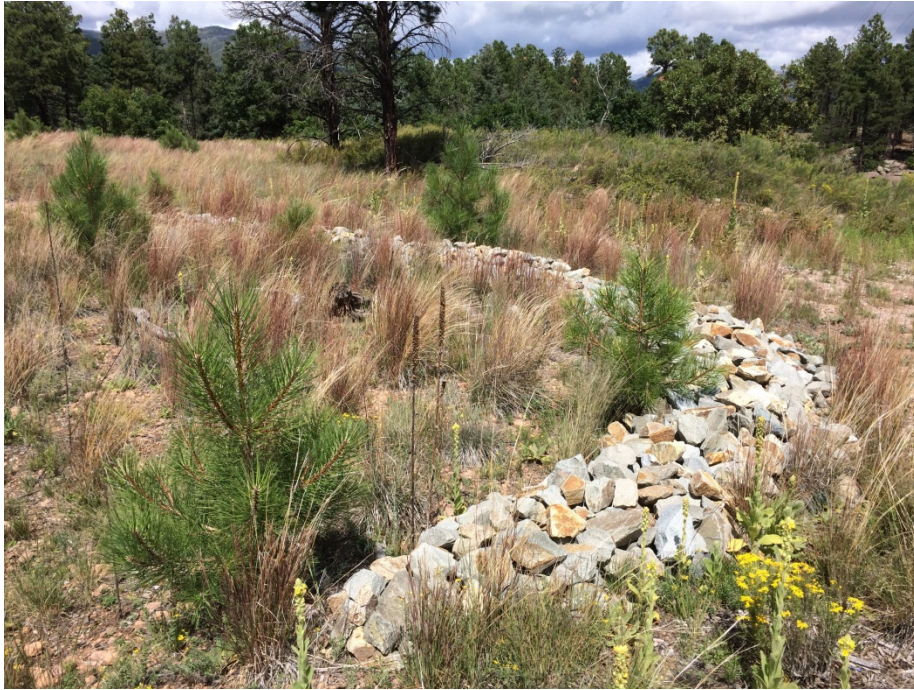
Figure 2 Rock berm (V00703120026—center of photo) at the top of drainage leading into Fishladder Canyon (September 2016). Note established vegetation. Condition of control: excellent.
