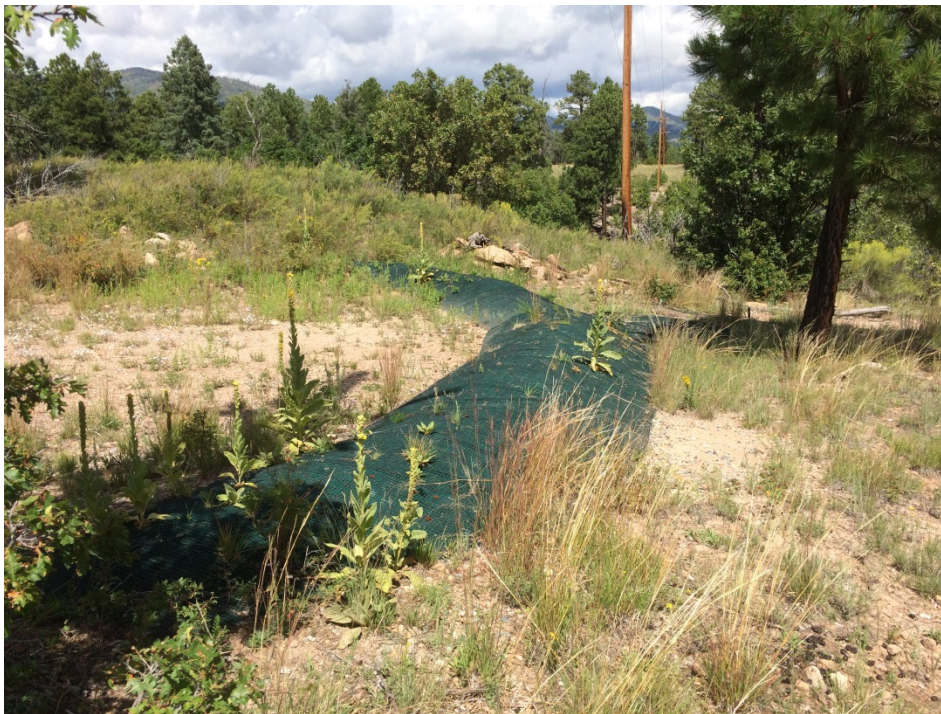
Figure 3 Earthen berm (V00703010027—center of photo) at the top of drainage leading into Fishladder Canyon (September 2016). Note established vegetation. Condition of control: excellent.
