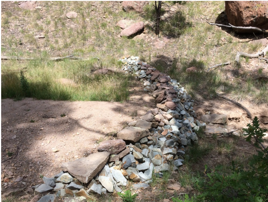
Figure 7 Rock check dam (V00706010024—center of photo) in Fishladder Canyon primary drainage (September 2016). Condition of control: very good.
