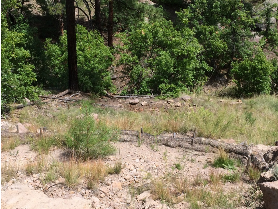
Figure 4 View downslope of the former fishladder location (September 2016). Note established vegetation above and below straw wattle (V007030600028–center of photo). Condition of control: good.
