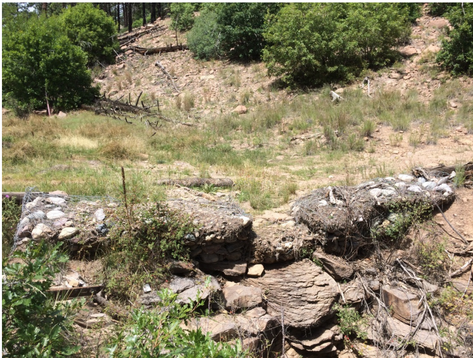
Figure 9 Gabion (V00707010002—center of photo) at access road crossing in Fishladder Canyon (September 2016). Note vegetation in channel upstream of control. Condition of control: good.
