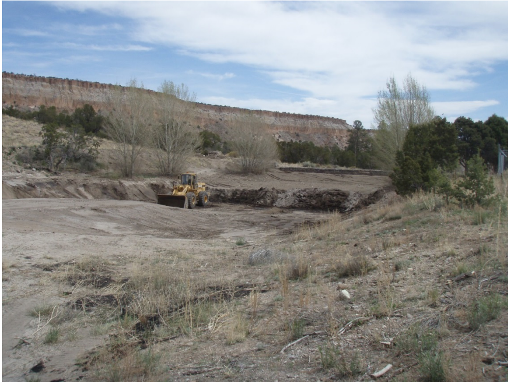
Figure B-8 Excavation of Los Alamos weir sediments in the lower basin in 2014
