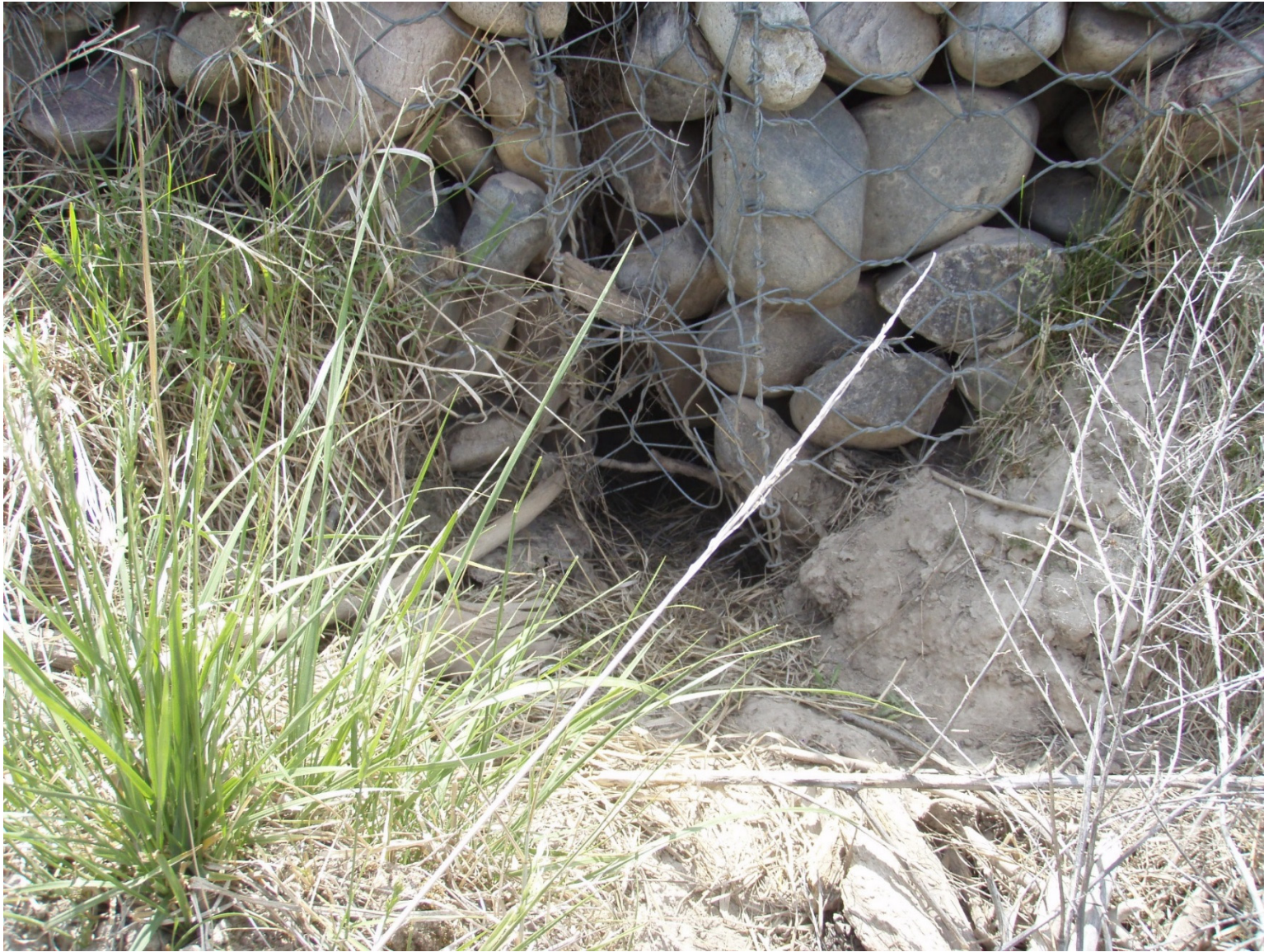
Photo 6 Los Alamos weir gabion structure at bottom of weir appearing to have undercutting
