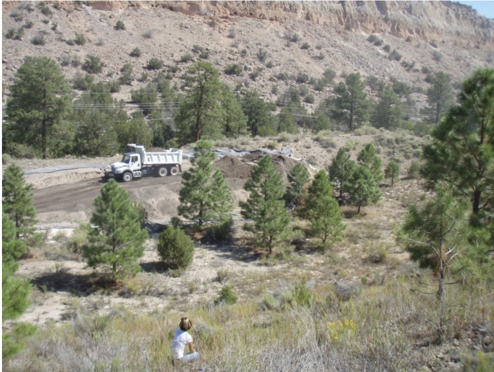
Figure B-4 Emplacement of excavated Los Alamos weir sediments in the borrow pit in 2012. The liner is visible around the sediments.
