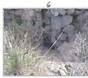
/mc_imageserver/entlan/WO/44555/Gabion at bottom of weir appearing to have undercu-image-2016-07-01T19-32-59.3000000Z.jpg
