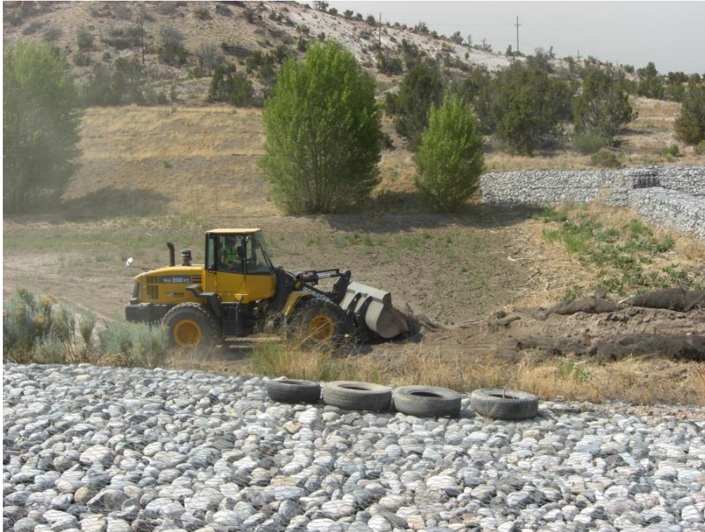
Figure B-1 Excavation activities within the Los Alamos low-head weir lower sediment basin in 2011
