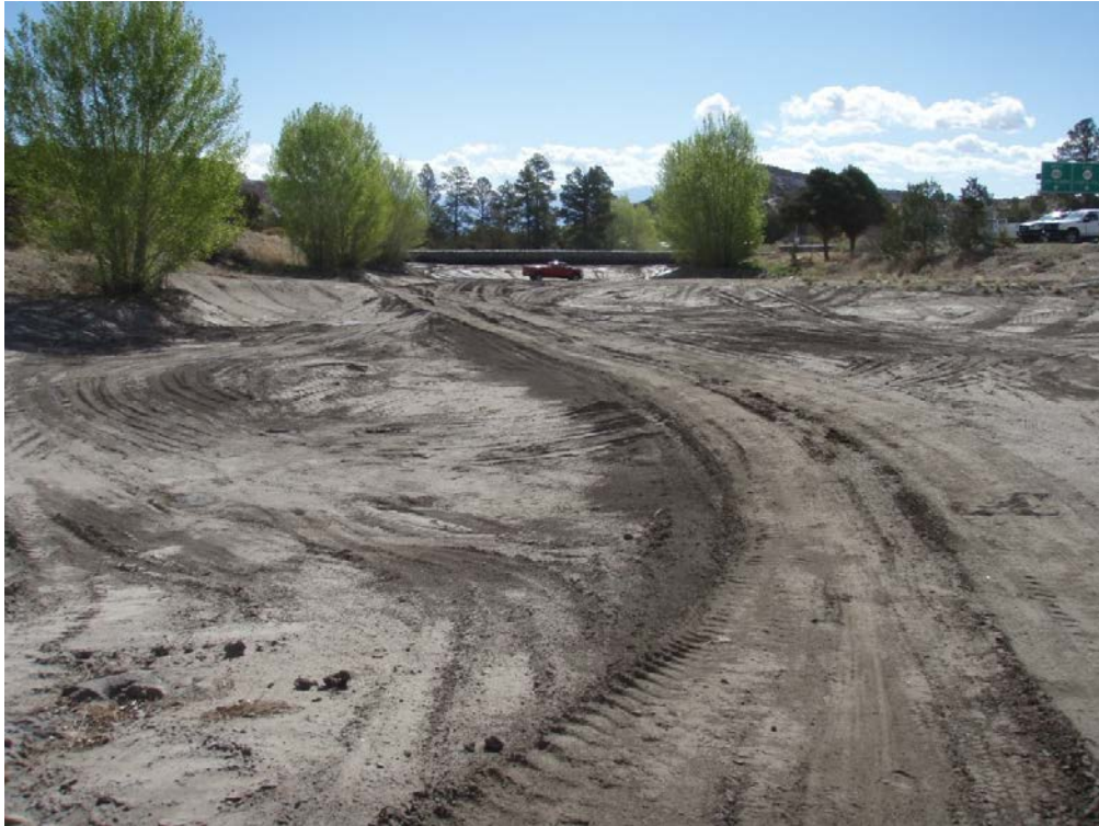
Figure B-6 Los Alamos weir lower basin after completion of 2013 excavation activities
