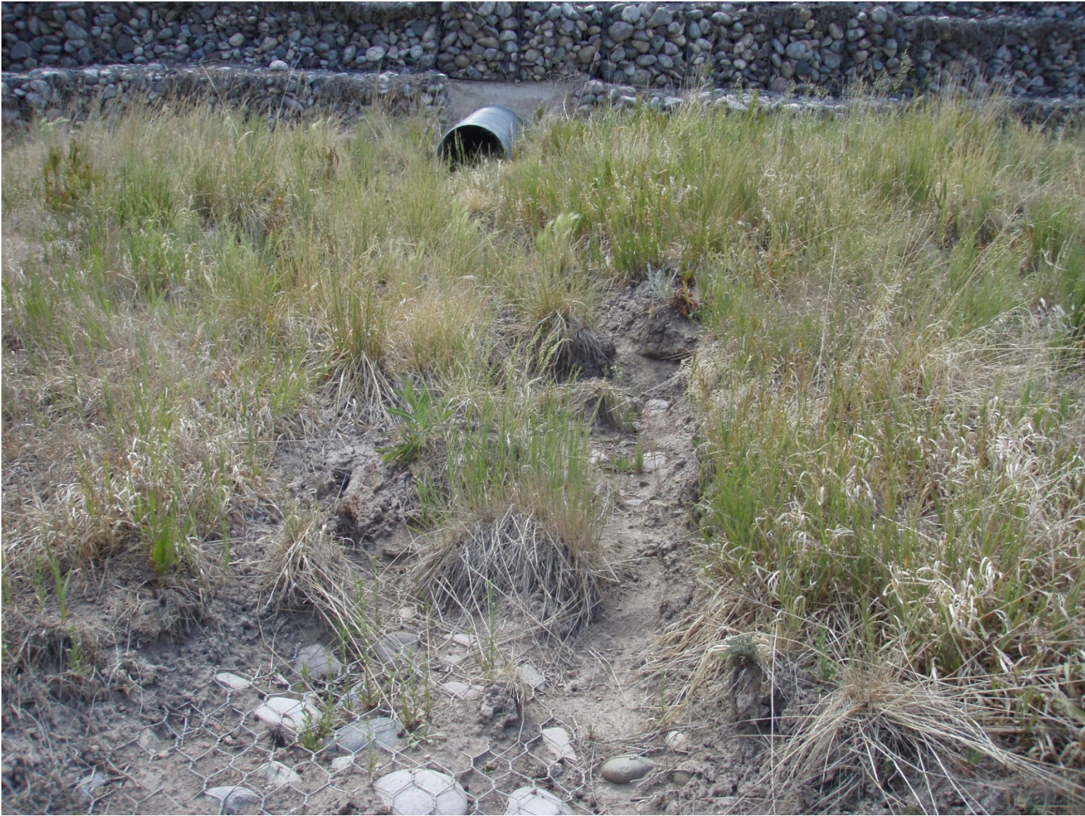
Photo 8 Downstream side of Los Alamos weir outlet pipe where erosion is occurring
