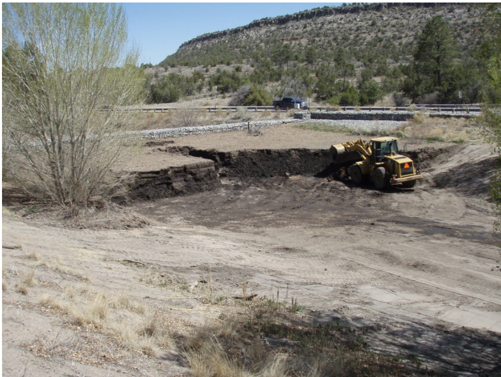
Figure B-5 Excavation of Los Alamos weir sediments in the lower basin in 2013
