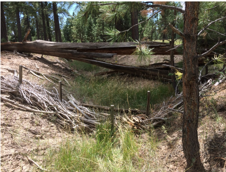
Figure 6 Juniper bale check dam located in drainage channel to 90s Line Pond, September 2016. Note vegetation in channel.
