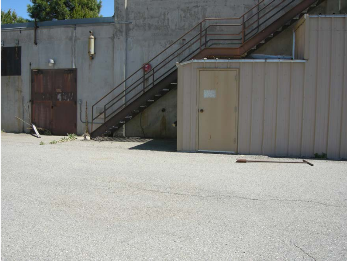
Figure C-3 Location of former underground tank AOC C-15-011, south of building 15-185, looking north
