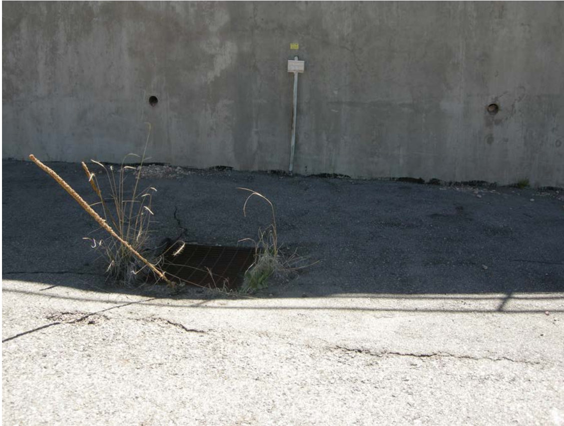
Figure C-2 Drop inlet at Solid Waste Management Unit (SWMU) 15-014(I) south of building 15-185, looking east
