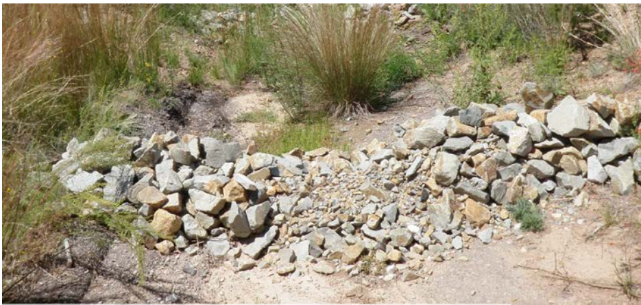
S-SMA-3.71, Rock Check Dam, S00806010008 (photo ID 8515-2)
