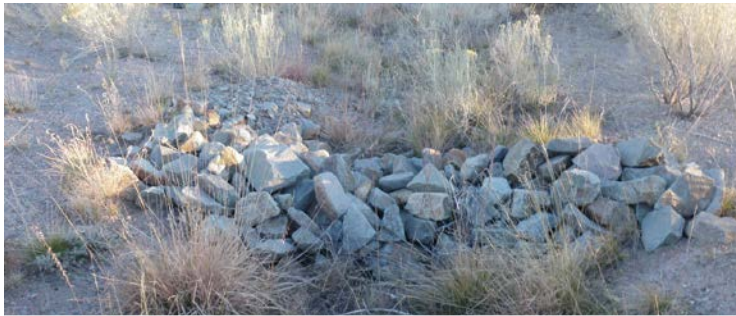
S-SMA-1.1, Rock Check Dam, S00206010008 (photo ID 29464-9)
