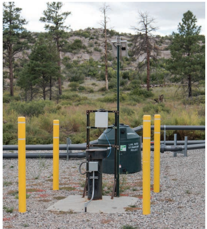
Well monitoring equipment on Laboratory property
