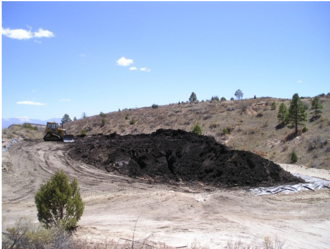
Figure 2 Excavated sediment being placed in former borrow pit in Los Alamos Canyon
