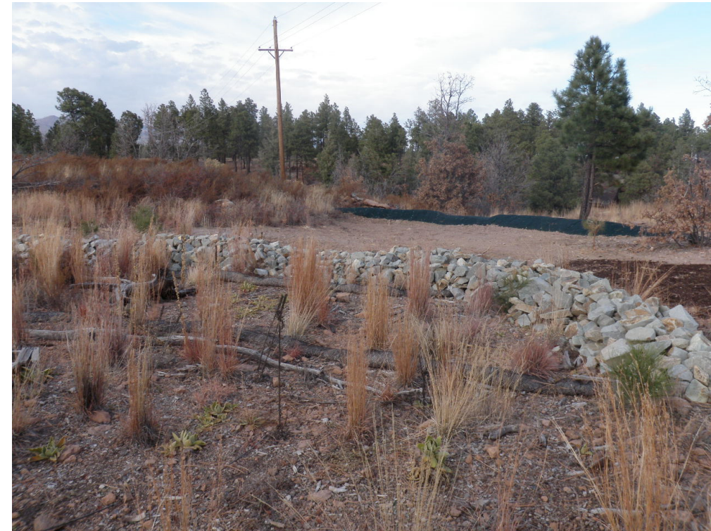
Figure 2 2014 Installation - Rock berm (V00703120026) and earth berm (V00703010027) at the top of drainage into Fishladder Canyon (11/14/2014)
