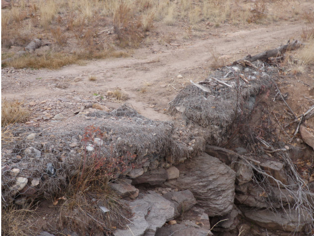
Figure 6 Gabion (V00707010002) at the crossing of the access road in Fishladder Canyon (11/14/2014)
