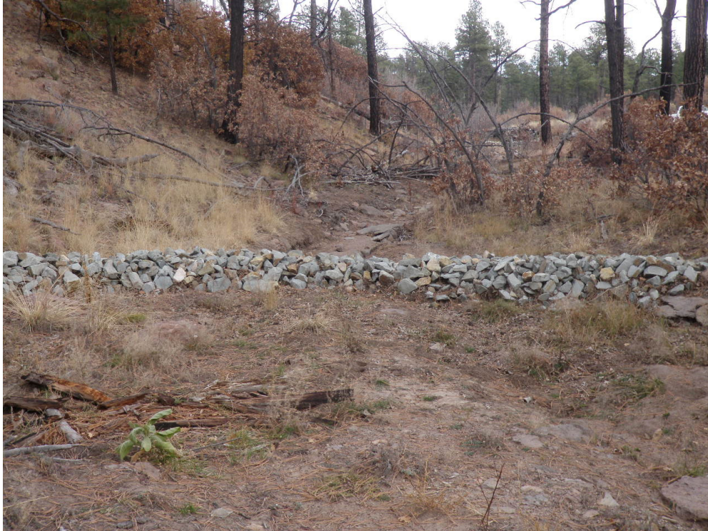
Figure 4 2014 Installation - Rock check dam (V00706010024) in the bottom of Fishladder Canyon (11/114/2014)
