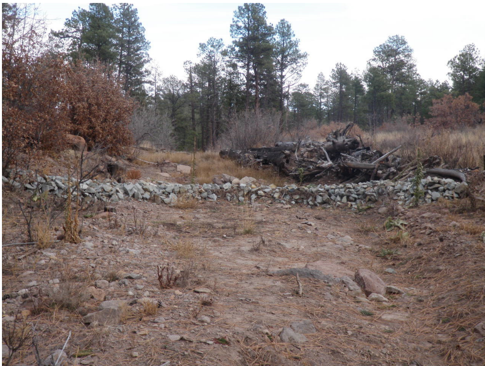
Figure 5 2014 Installation - Rock check dam (V00706010025) in the bottom of Fishladder Canyon (11/14/2014)
