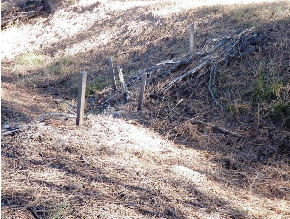
Figure 3 Juniper bale check dam in channel draining to 90s Line Pond, November 2014
