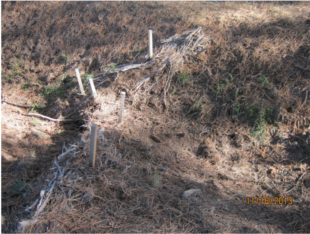
Figure 3 Juniper bale check dam in channel draining to 90s Line Pond, November 2013
