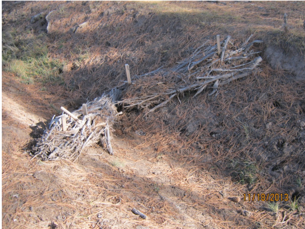
Figure 1 Juniper bale check dam in channel draining to 90s Line Pond, November 2013
