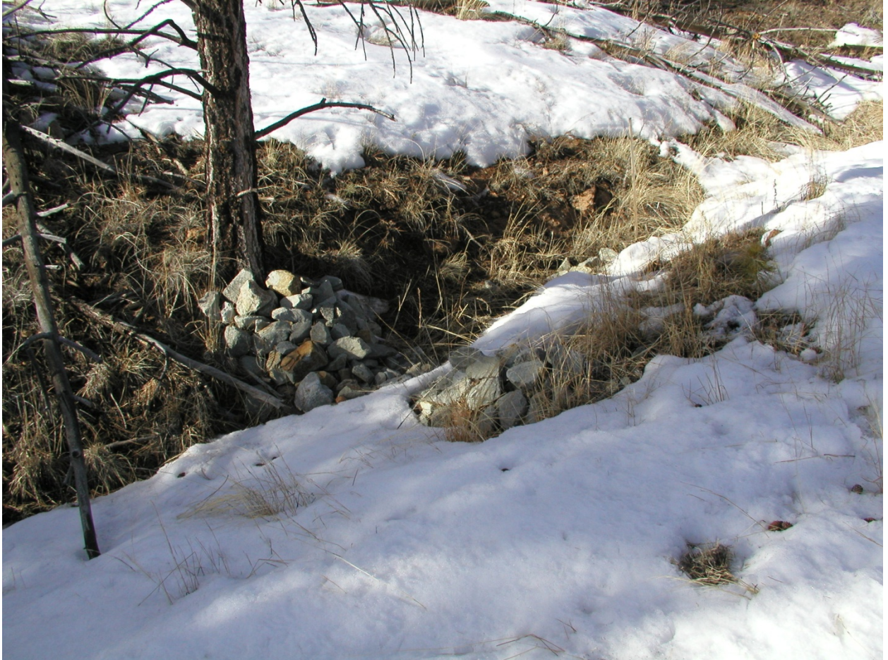
Figure 4 Damaged rock check dam
